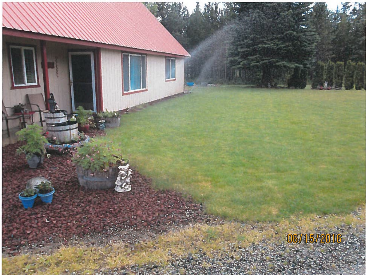
Automatic irrigation sprinklers in from of house.
