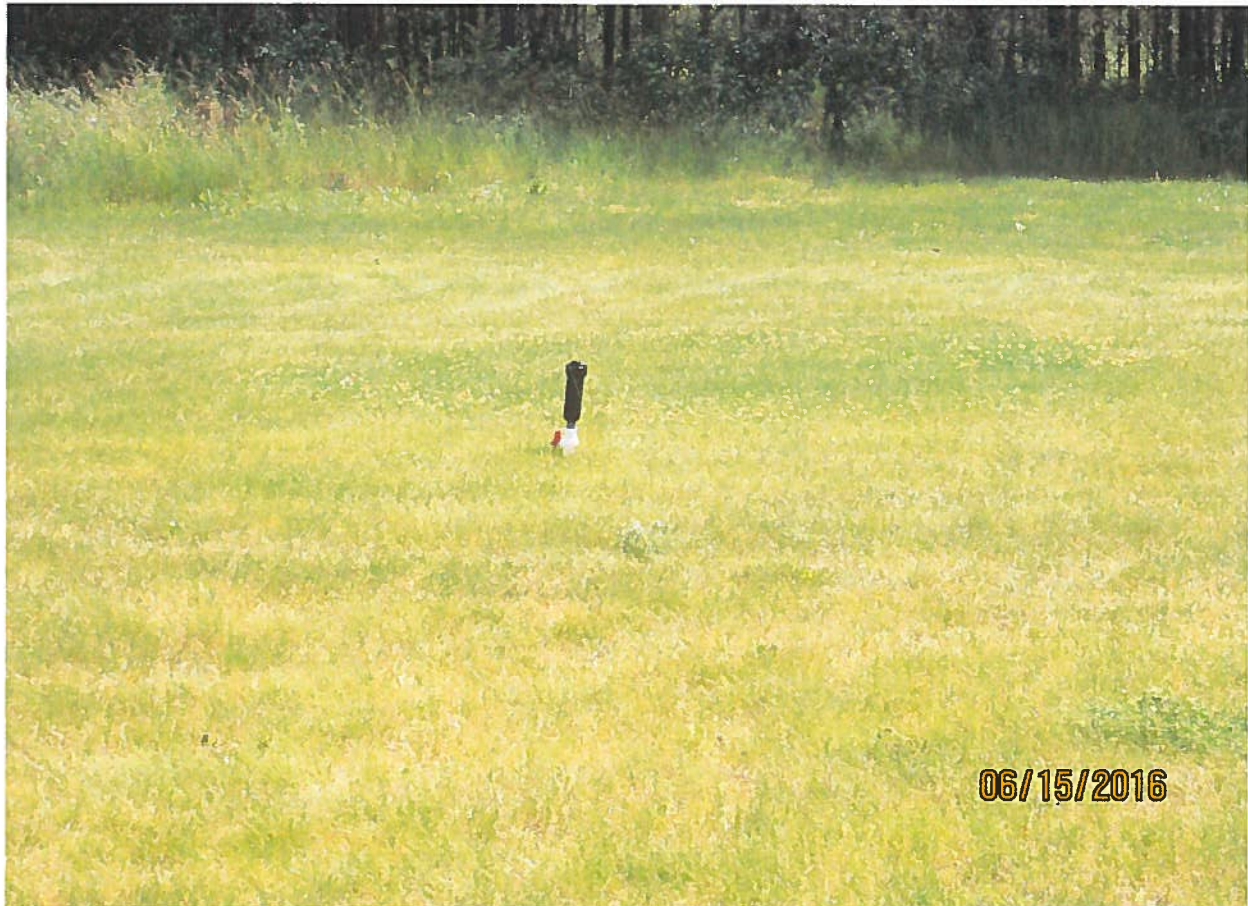
Irrigation sprinkler along driveway.
