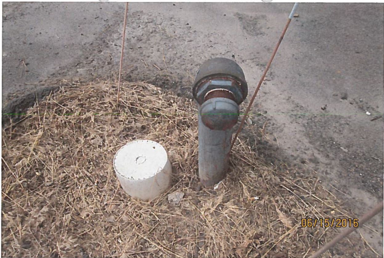
Fire protection hydrant.
