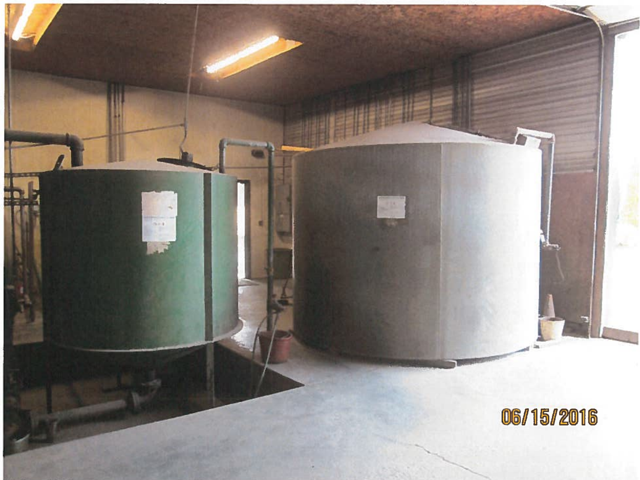
Tanks where water would be pumped from well and then mixed with chemicals to be sprayed on timber products.
