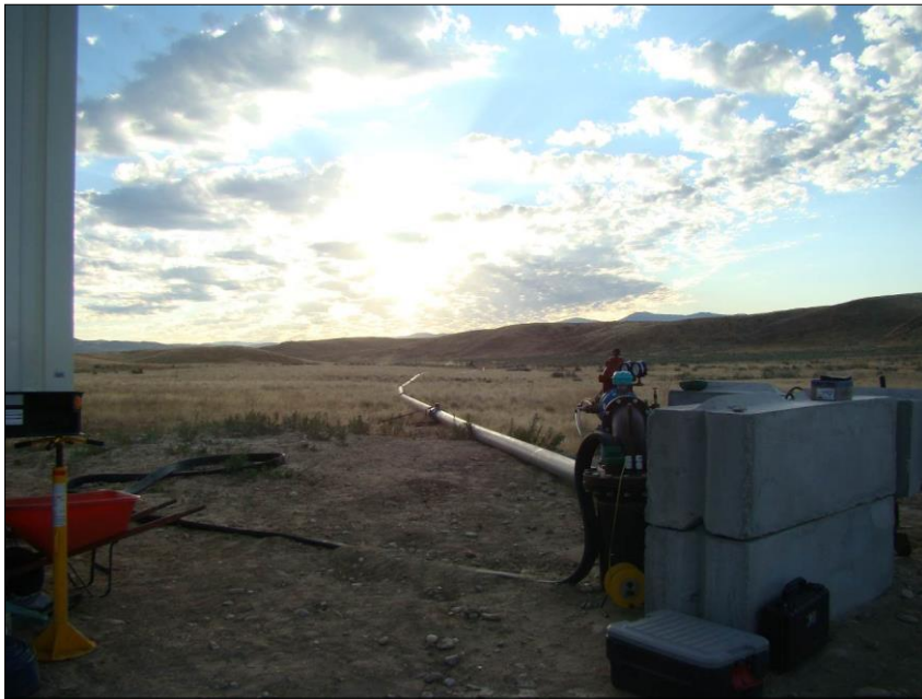
7-17-2016 – Aquifer test discharge routed through ~1,800' of 10" Victolic clamped pipe with seventeen 4" discharge outlets along pipeline spreading water over large areas to prevent water from going to farmer's fields.
