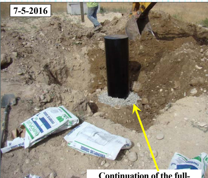
Continuation of the full-depth annular well seal around the municipal well head using chipped bentonite clay around casing.
