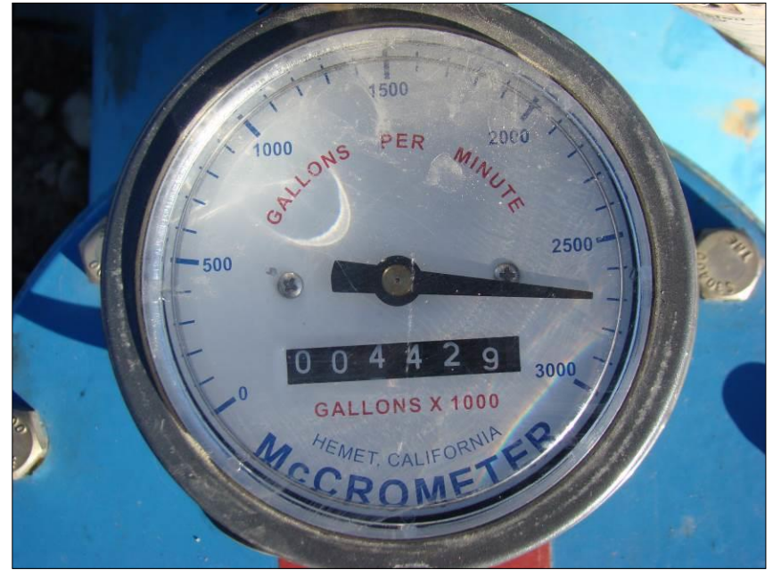
2-23-2016 – Flow-meter registering 2,700 gallons/minute during first day of 80-hour long aquifer test of Spring Valley Municipal Well #1. At end of test, totalized flow matched the instantaneous readings and pumping time.
