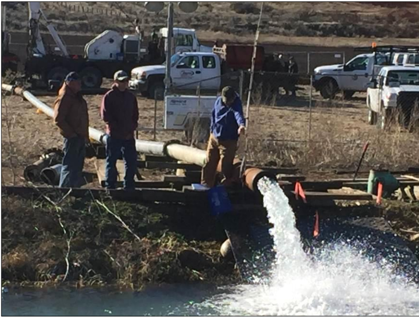
2-22-2016 – Well development and aquifer test discharge using a circular orifice weir to measure flow. Ken Acuff and his staff of the City of Eagle Water Department visit site during test.
