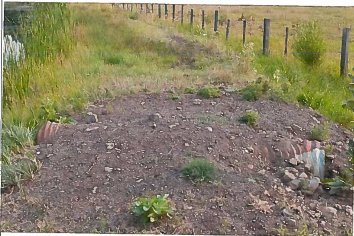
Photo 5 is further south and is located in the small adjacent pond. The fence line is border between Whitney and Raney Ranches. This is the overflow from the 2 ponds which goes to the Raney Ranch. There is no weir or anything other than the pipe.
