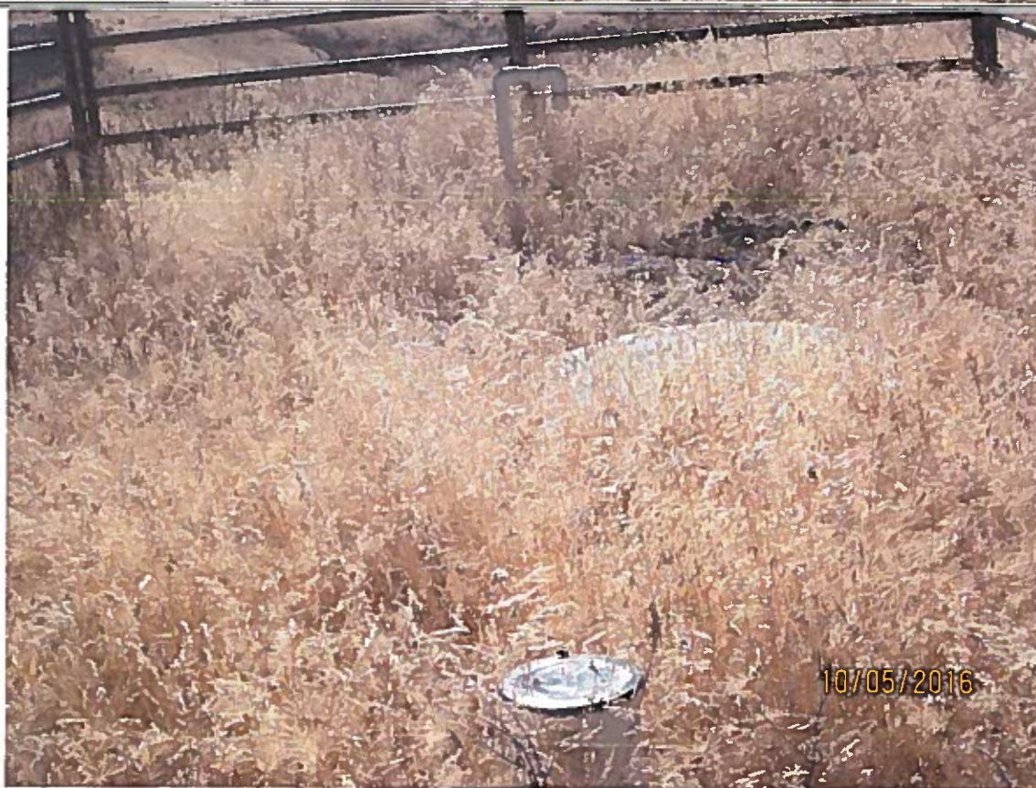
Riser and buried 1,050 gallon storage tank for domestic use.
