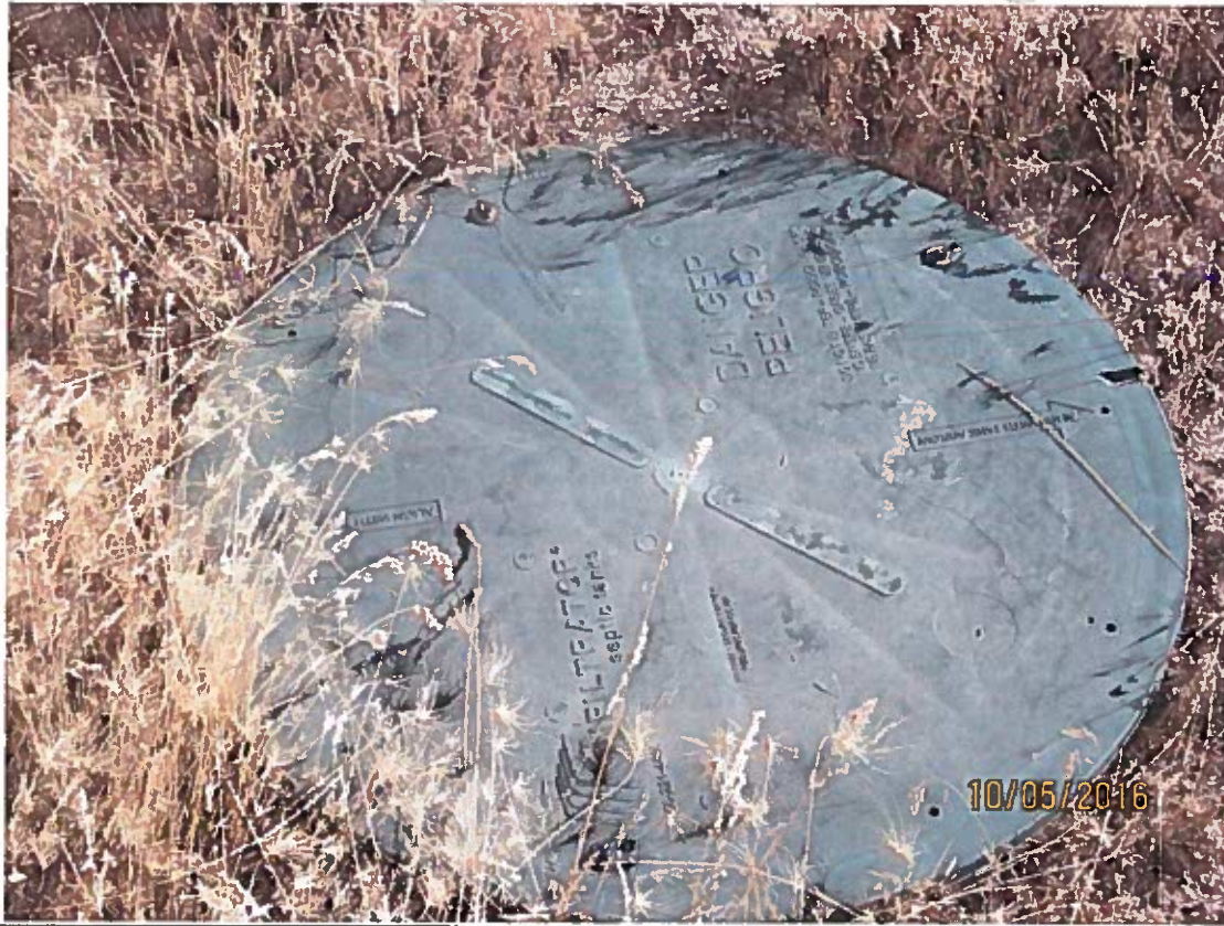
Buried 1,050 gallon water storage tank.
