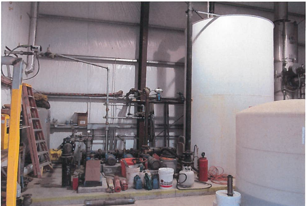
Water distribution room.
