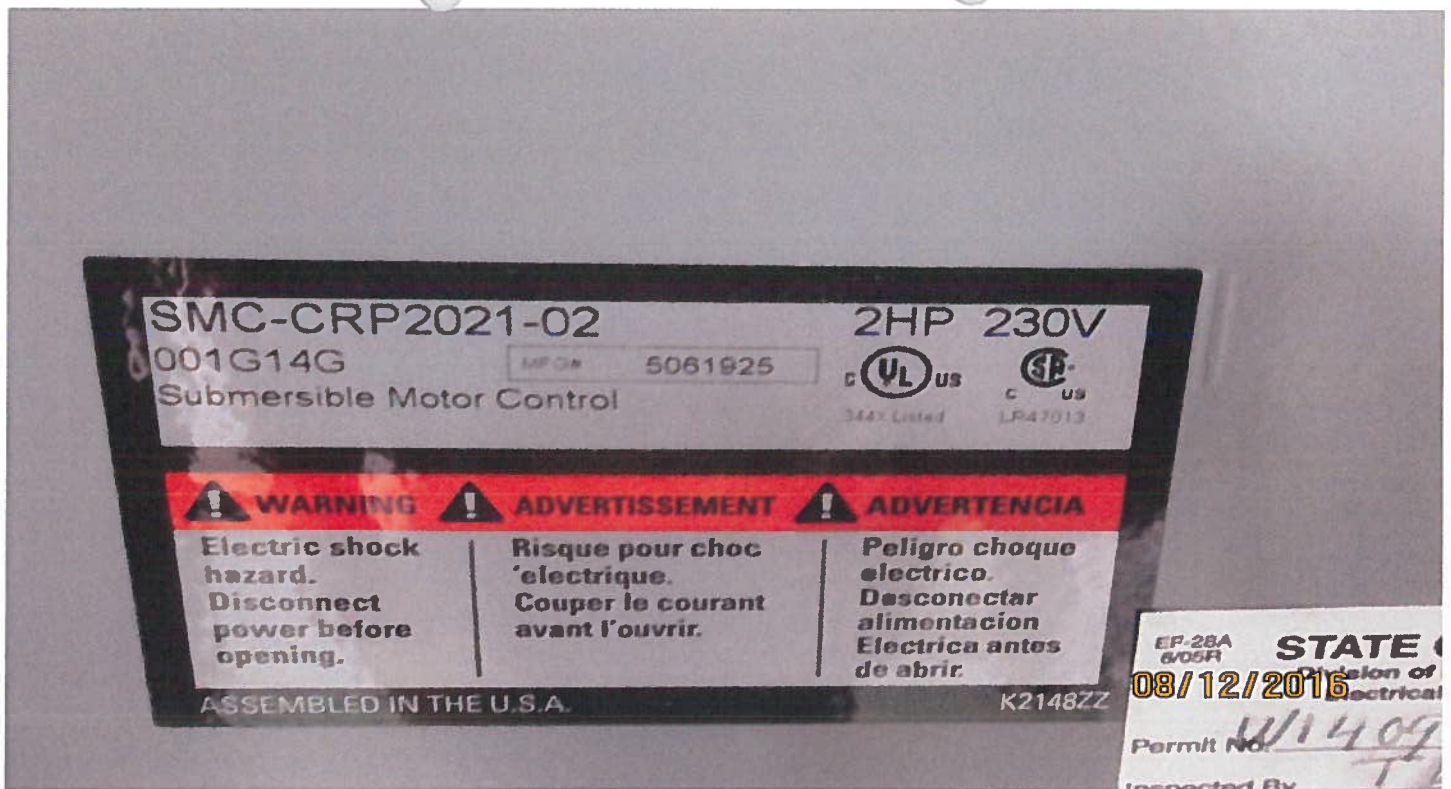
Well control box in fire station. 2 hp pump.
