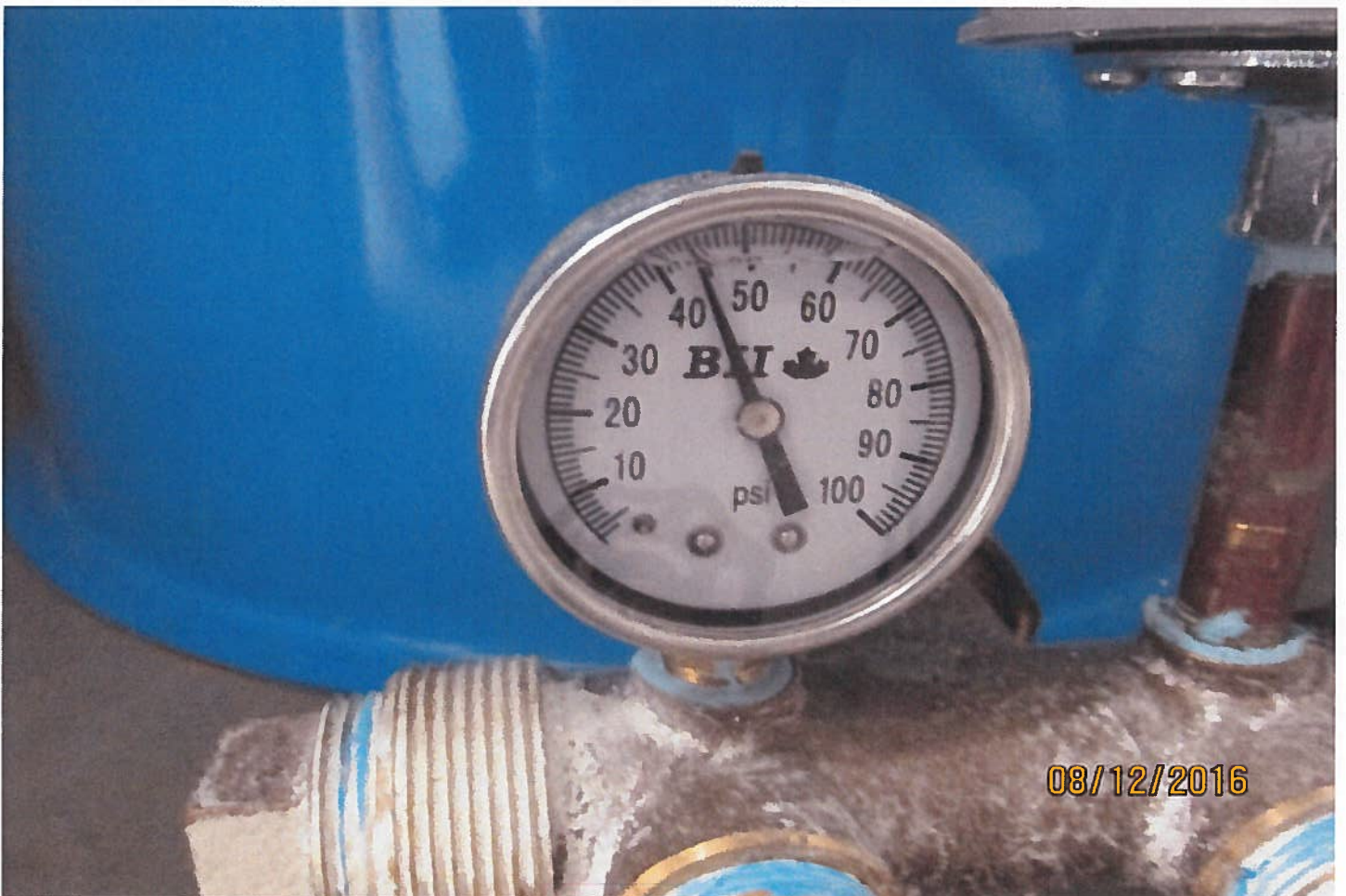
System running at 45 psi.
