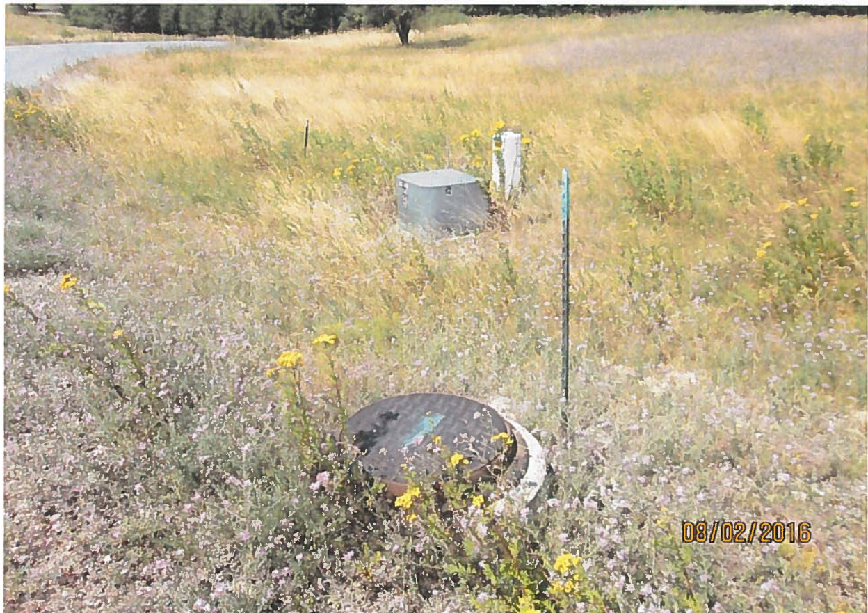
Sewer, water, and electric lines.
