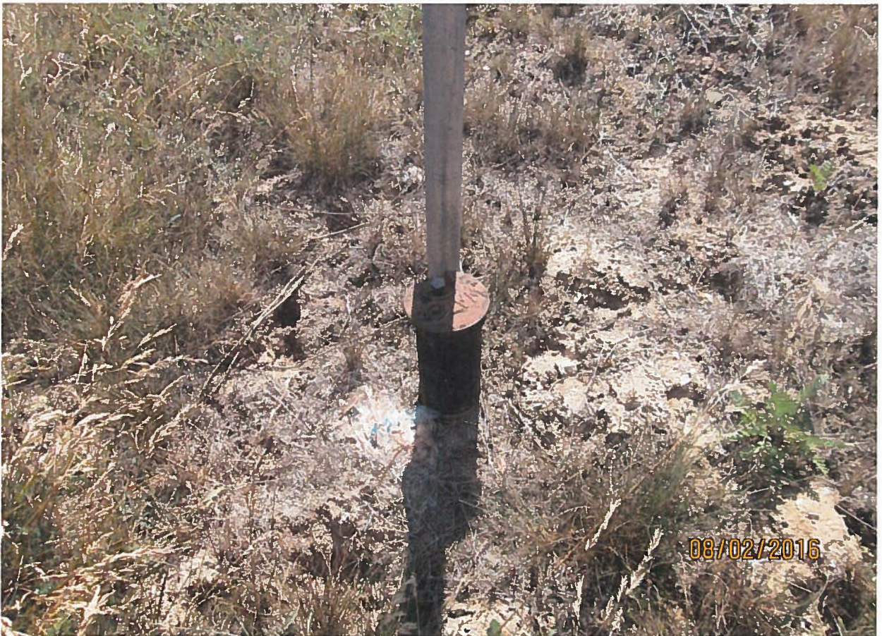
Various water stub-in along road.
