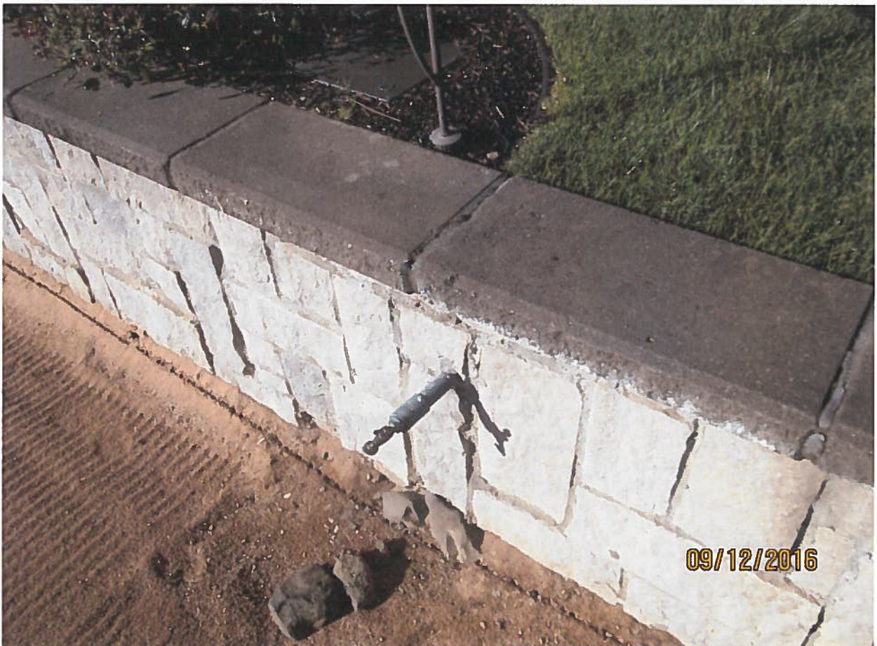
Irrigation mainly by automatic sprinklers, but hydrants located around property as well.
