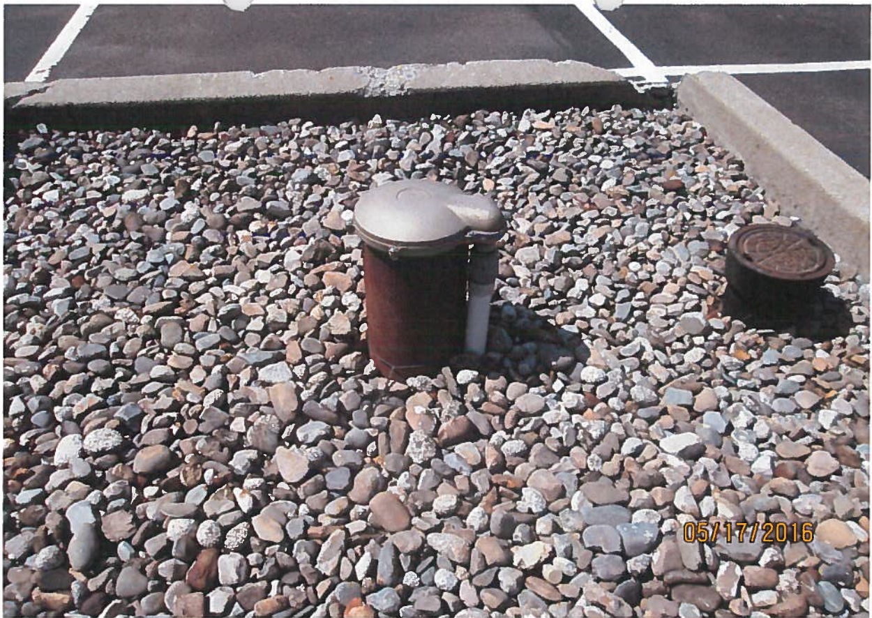
Well #2. Only well serving marina. 3hp pump with maximum pumping capacity at 45 gpm.
