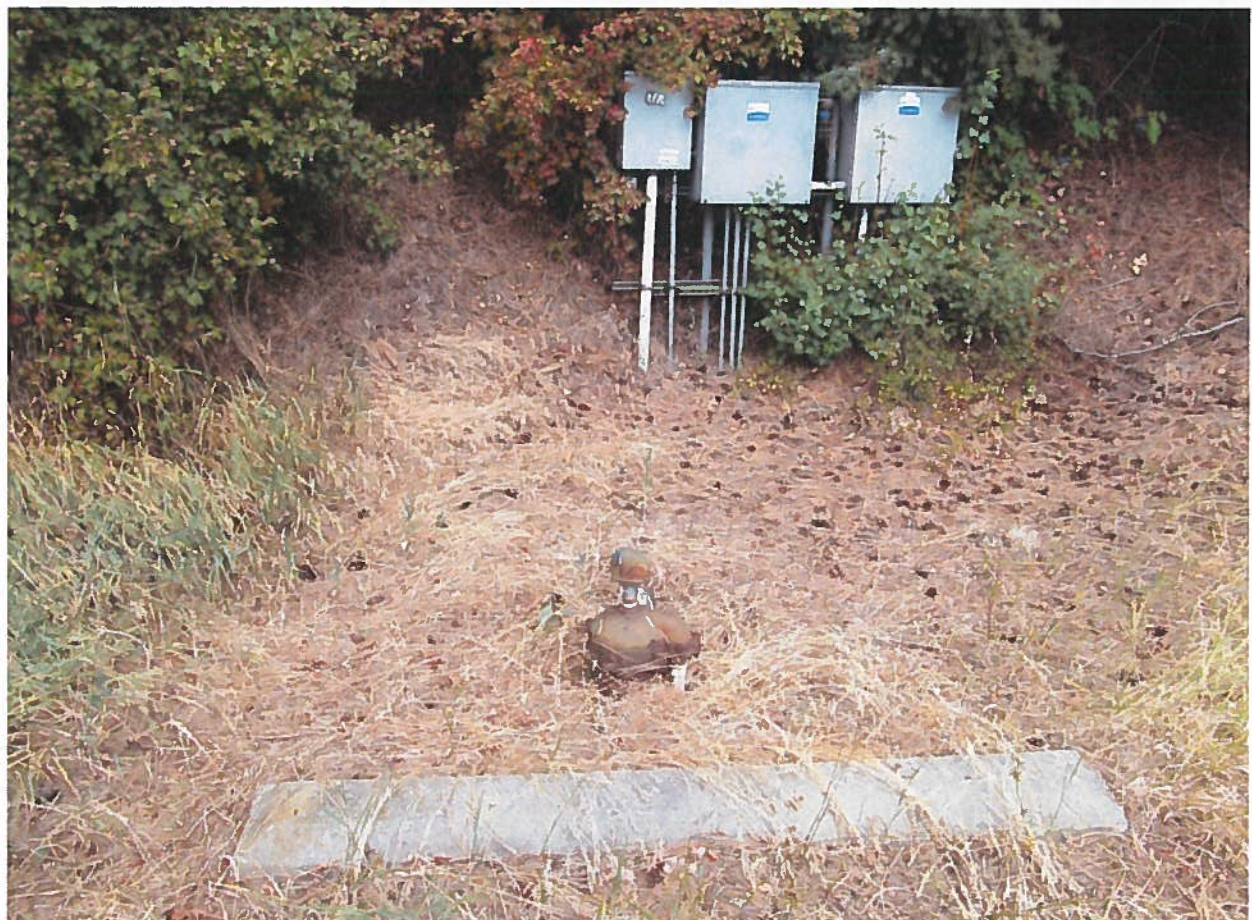
Well #1. Currently not being used because of sediment issues.
