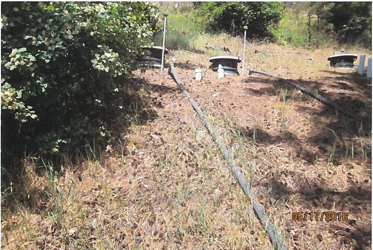
Storage tanks on hill above Well #1.
