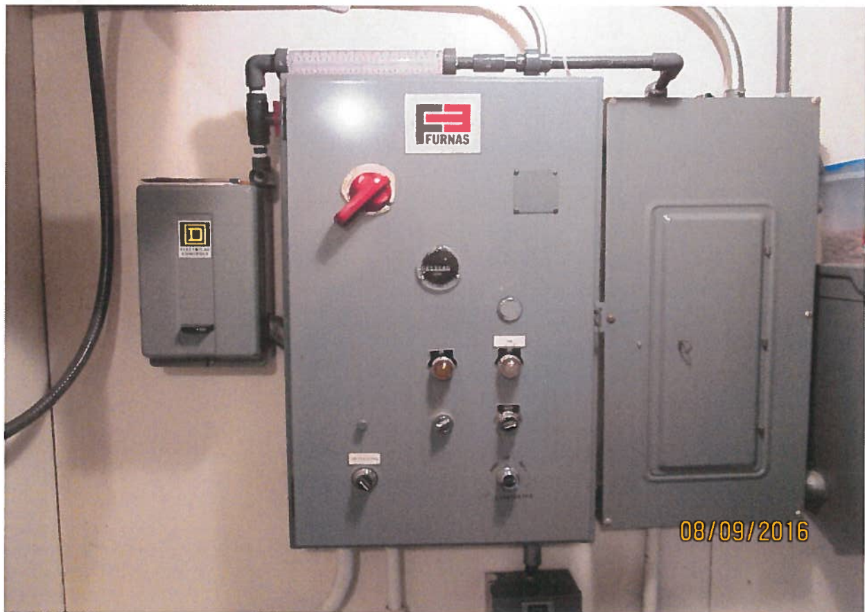
Control panel for all pumps.
