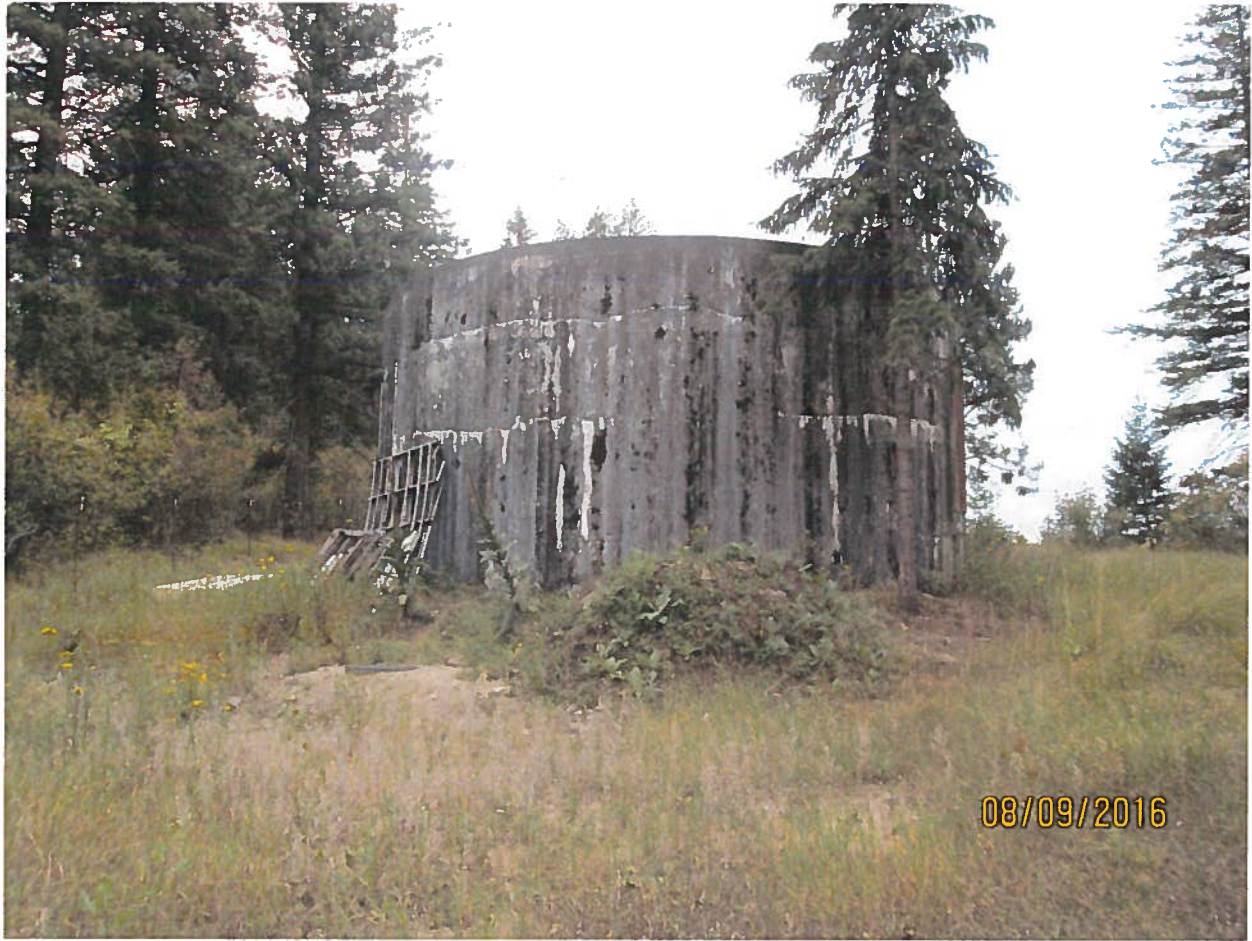
100,000 gallon reservoir at top of hill above service area.
