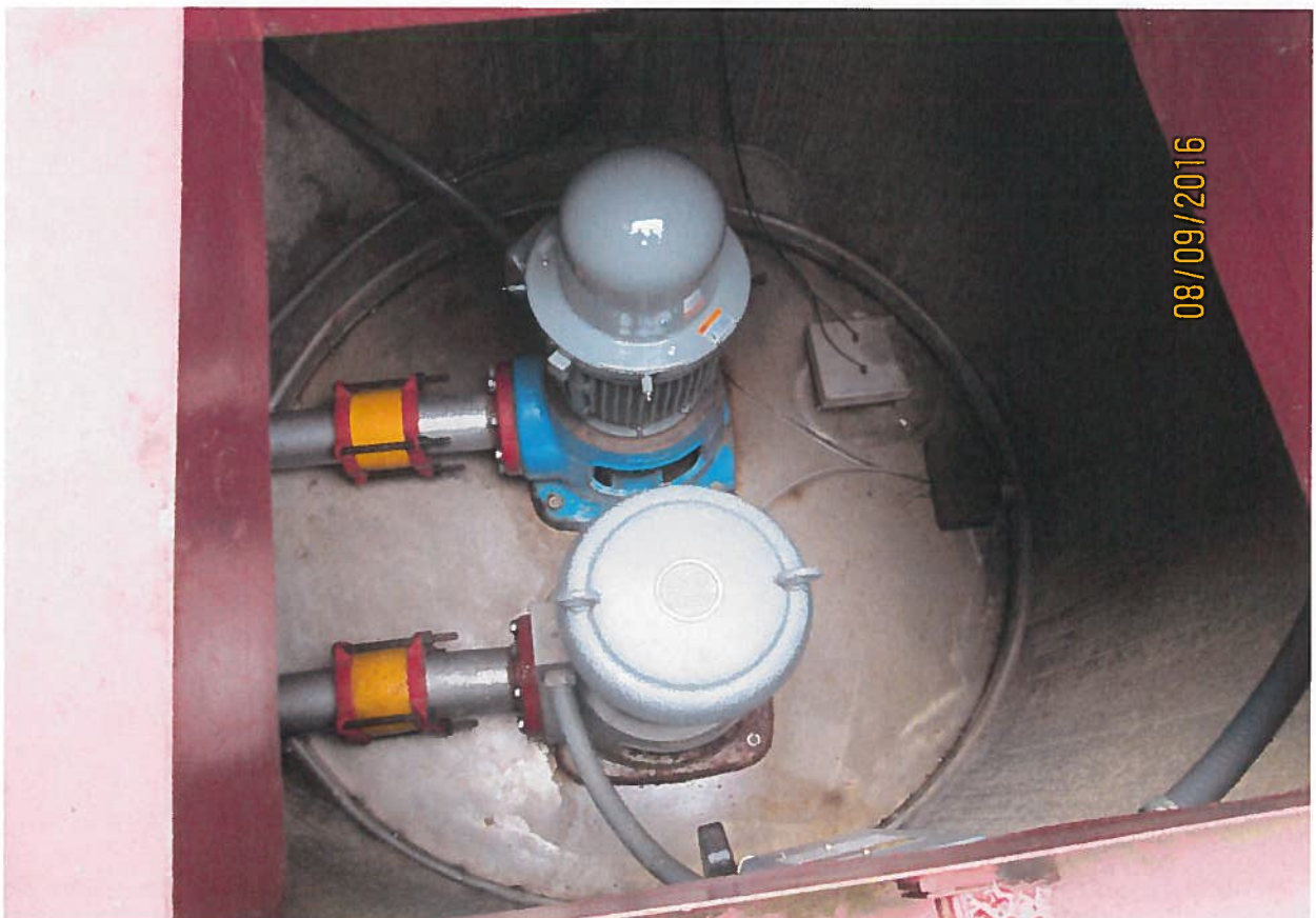
Looking down at both pumps in the spring source (96-7113)
