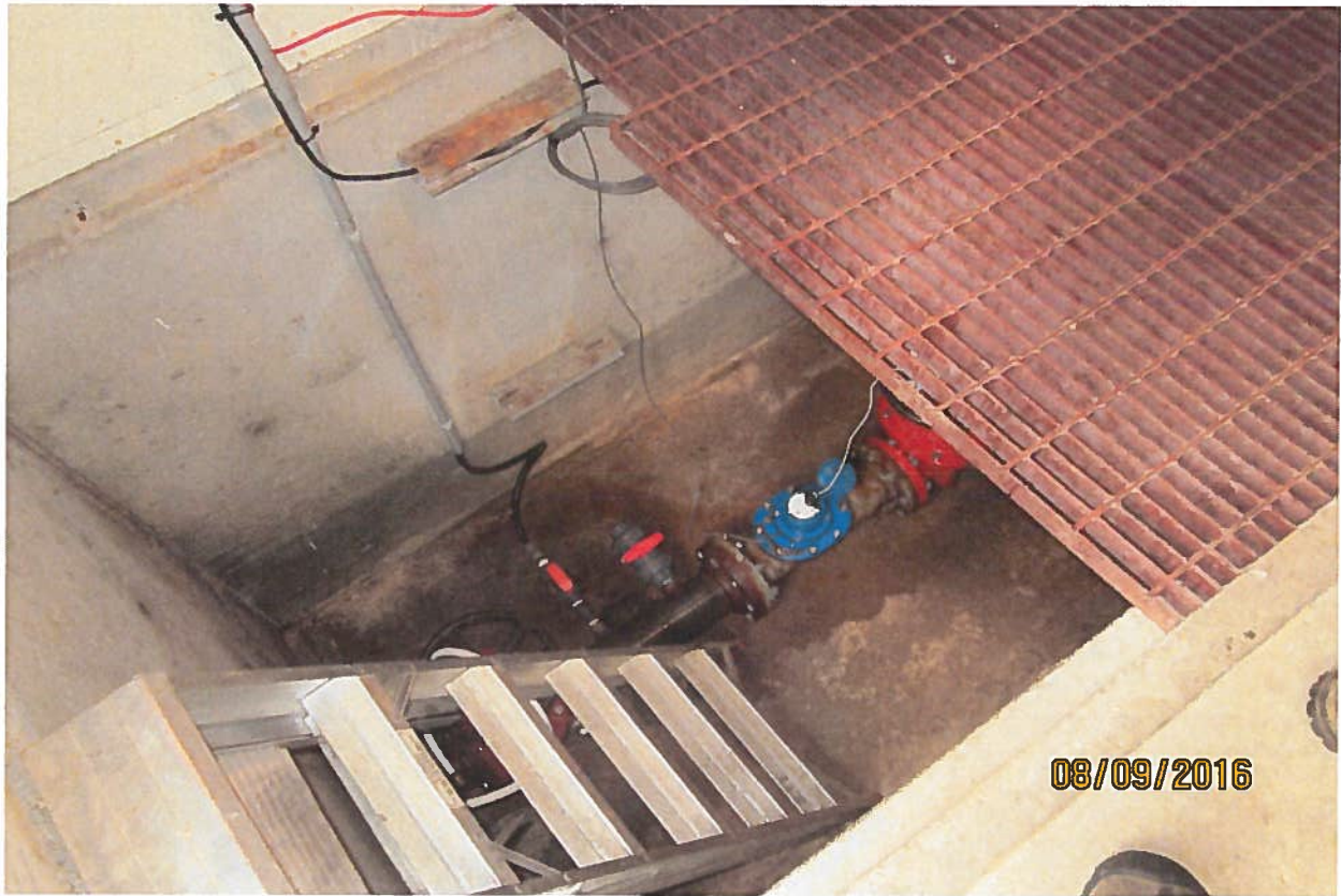
Meter on system after both well and spring sources are combined.
