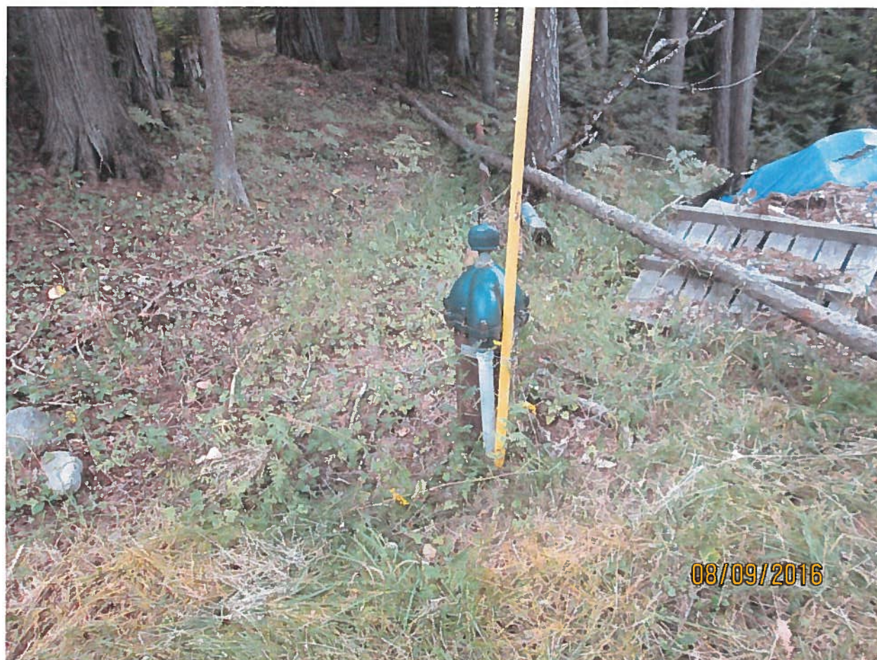
Well 96-95-N-174. 15hp pump set at 65 feet.
