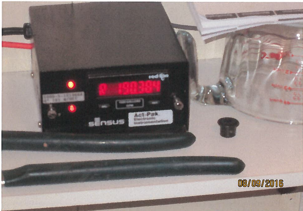
Flow meter on system when well was only source pumping water.
