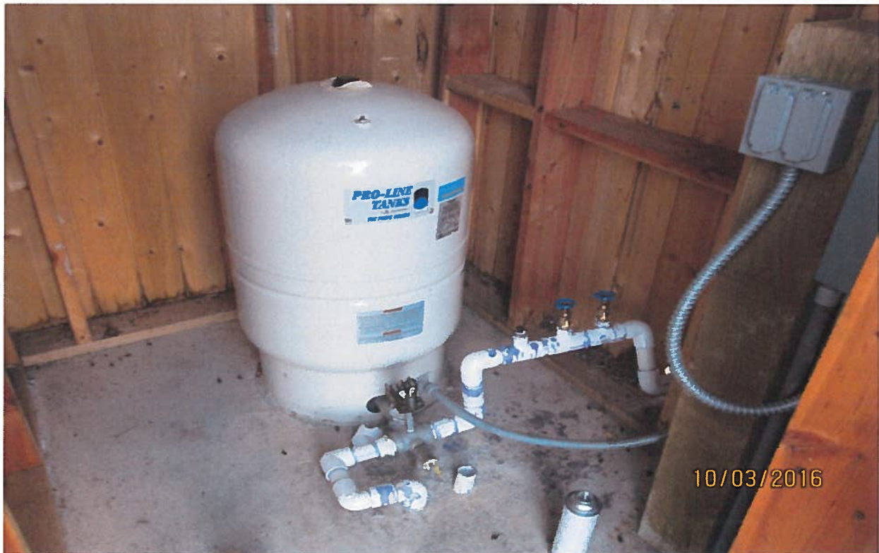
Pump house near shore with pressure tank to deliver water for irrigation.
