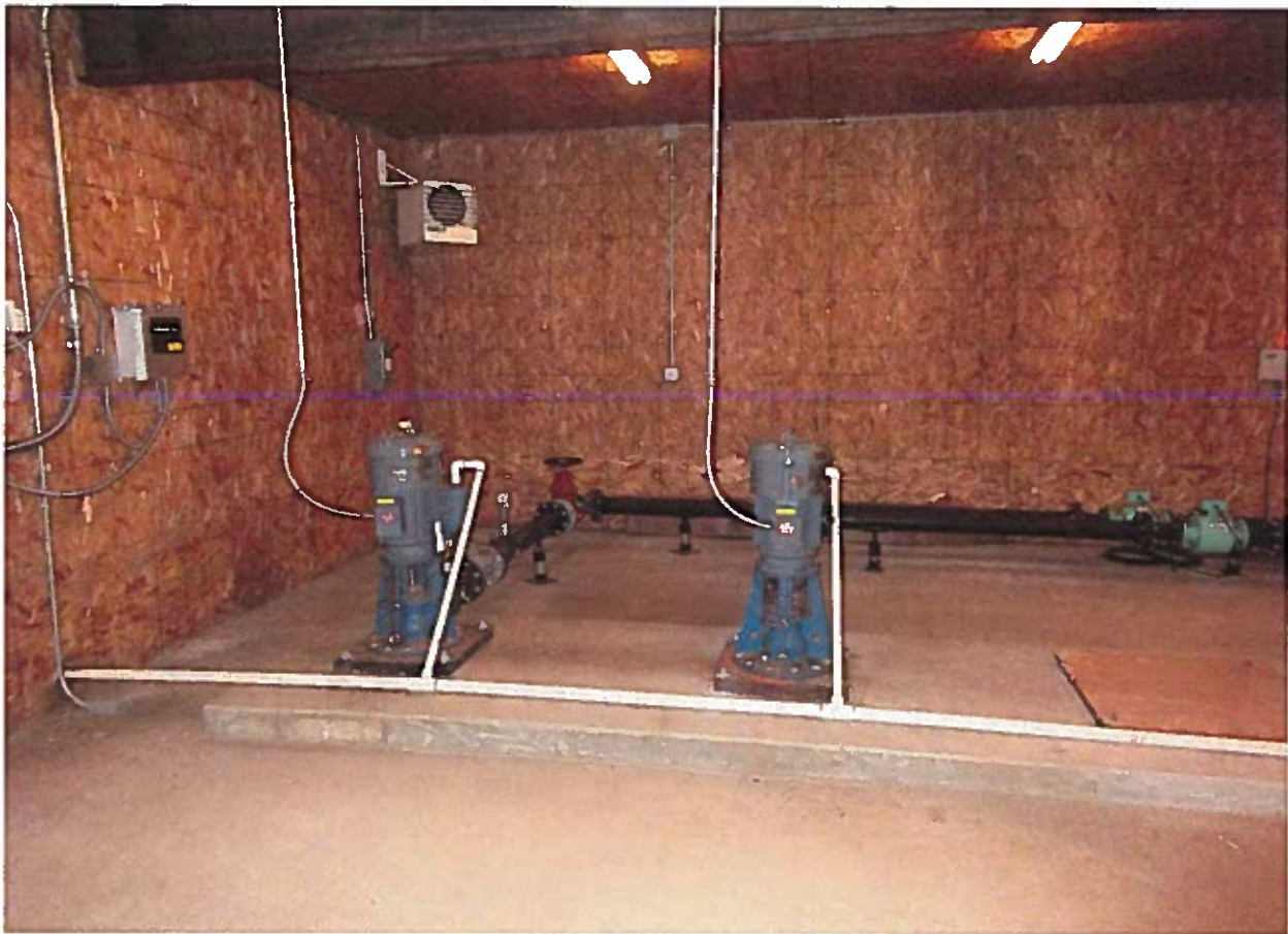
Inside pump house for fire protection in neighboring subdivision, Driggs Centre, looking at two of three pumps
