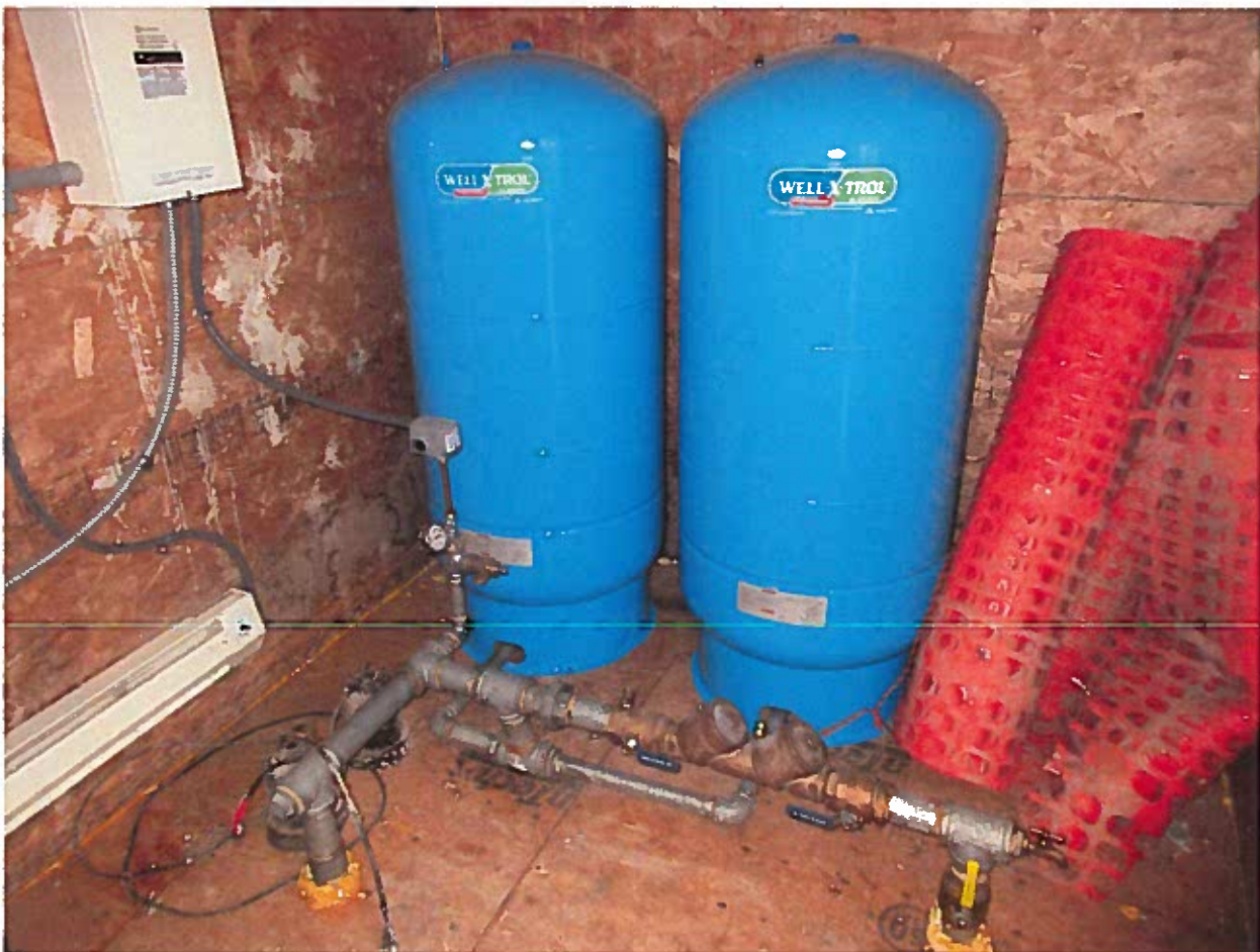
Inside pump house looking at the two pressure tanks.
