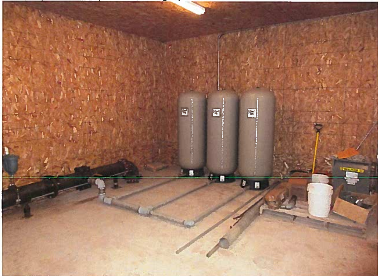
Inside pump house for fire protection, looking at pressure tanks
