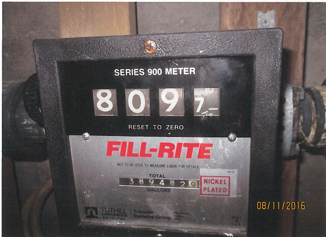
Flow meter on system.
