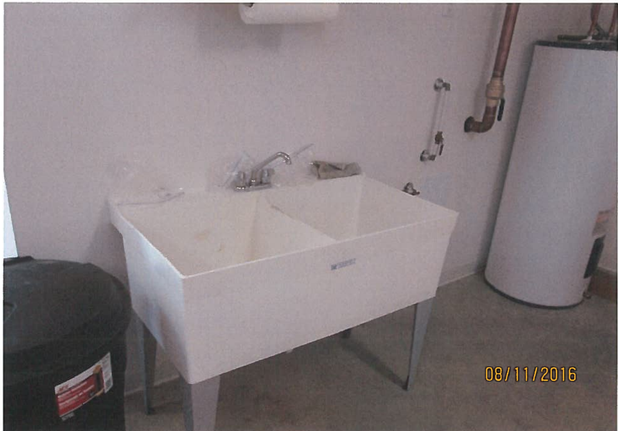
Sink and hot water heater for fire station.
