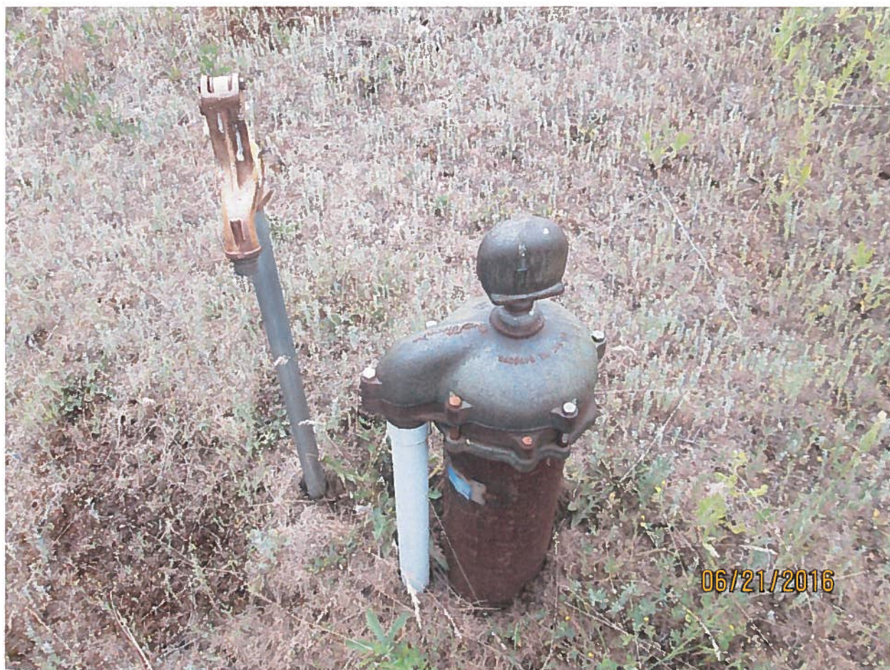
Well D0003185 given IDWR tag A0015432. Unknown pump size, 5 gallon bucket showed 25 gpm.
