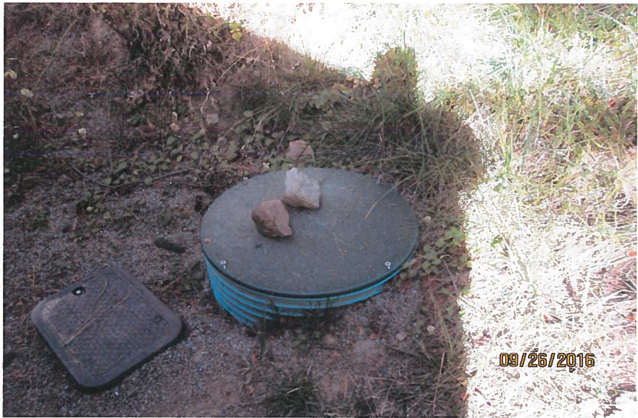
1,000 gallon cistern on system.
