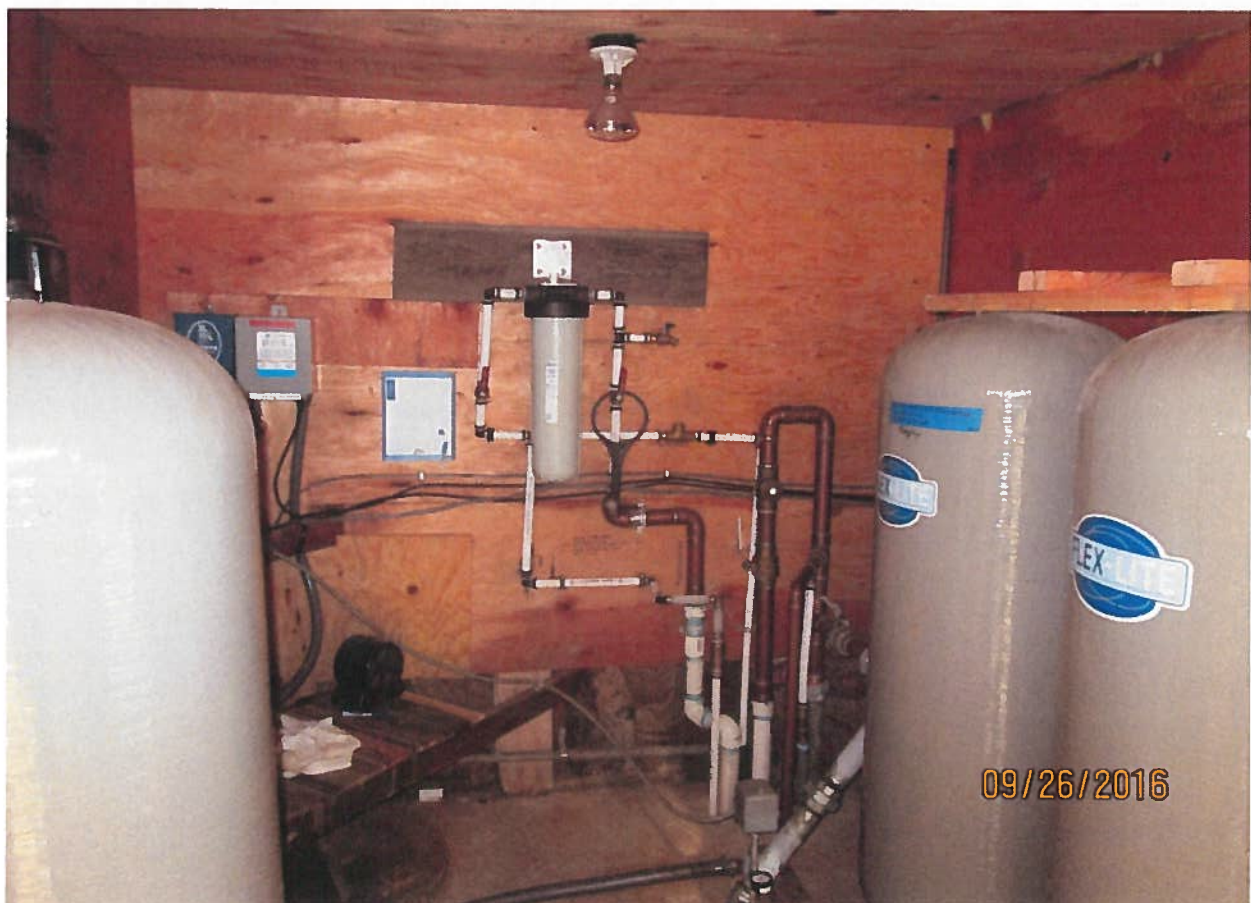
Inside pump house where water from Lake Coeur d' Alene and well are mixed together.
