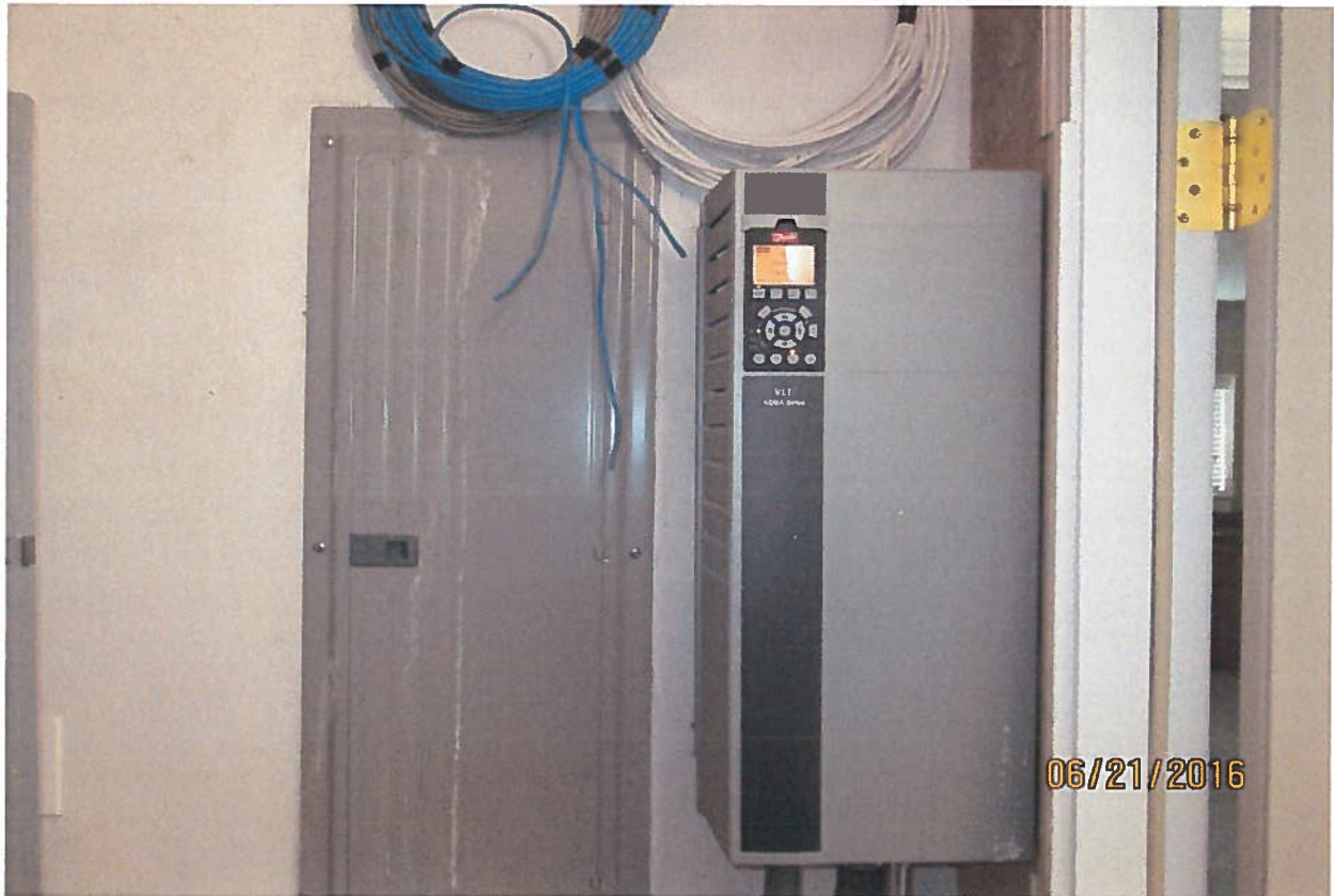
Danfoss VLT AQUA DRIVE tells us well has a 25hp pump. Applicant also said he put in 25hp pump.
