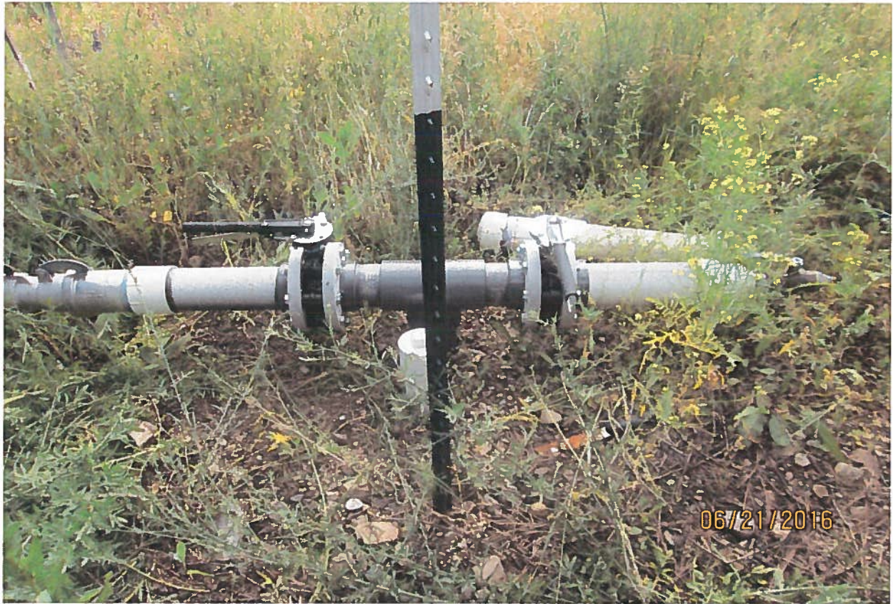
Buried main line with risers like this every 100 feet.
