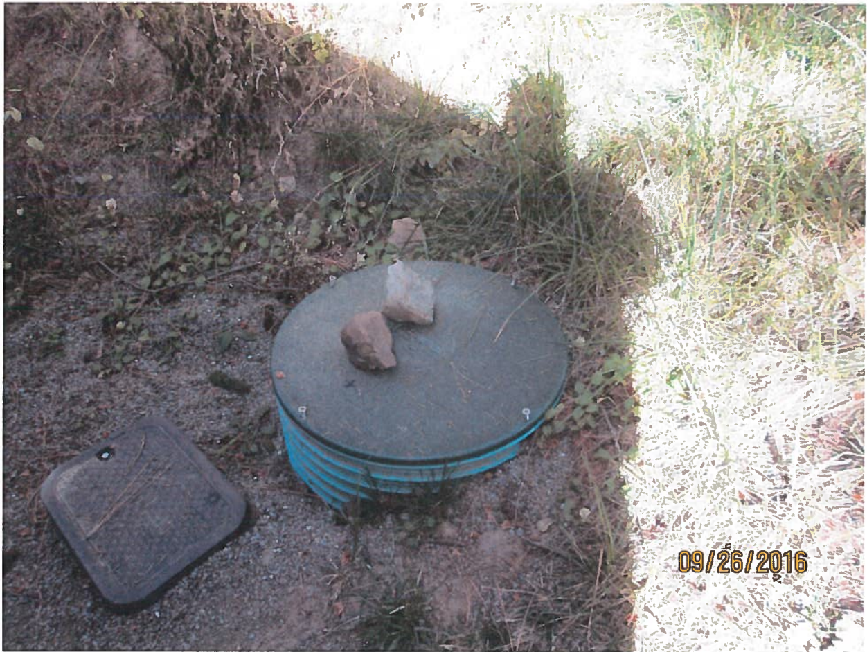
1,000 gallon cistern on system.
