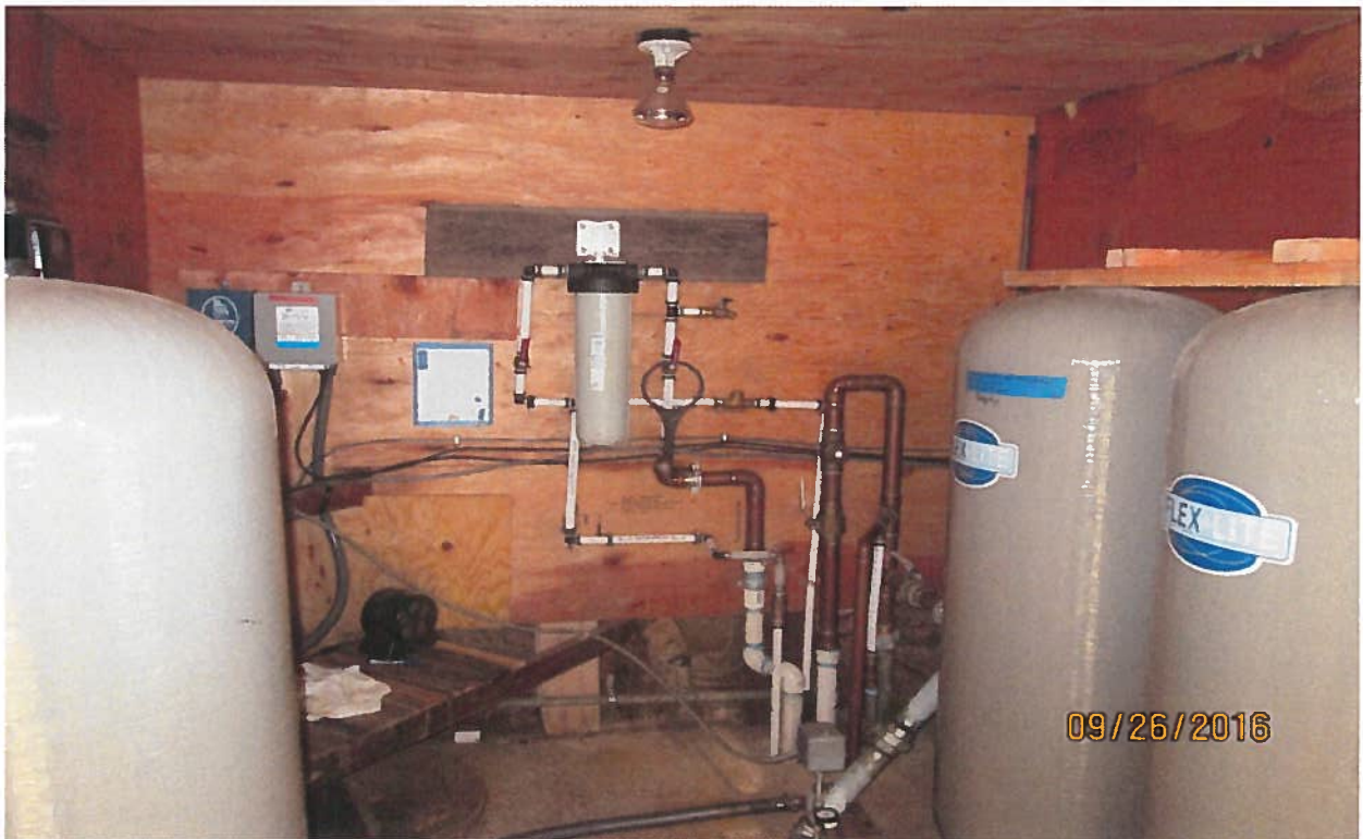
Inside pump house where water from Lake Coeur d' Alene and well are mixed together. 95-15125 and 95-15124 covers applicant from both sources.
