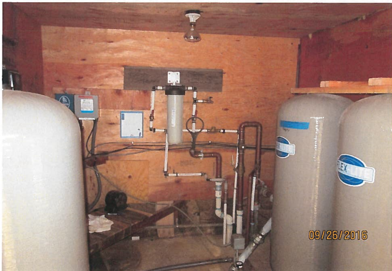
Inside pump house where water from Lake Coeur d' Alene and well are mixed together. 95-15125 and 95-15124 covers applicant from both sources.
