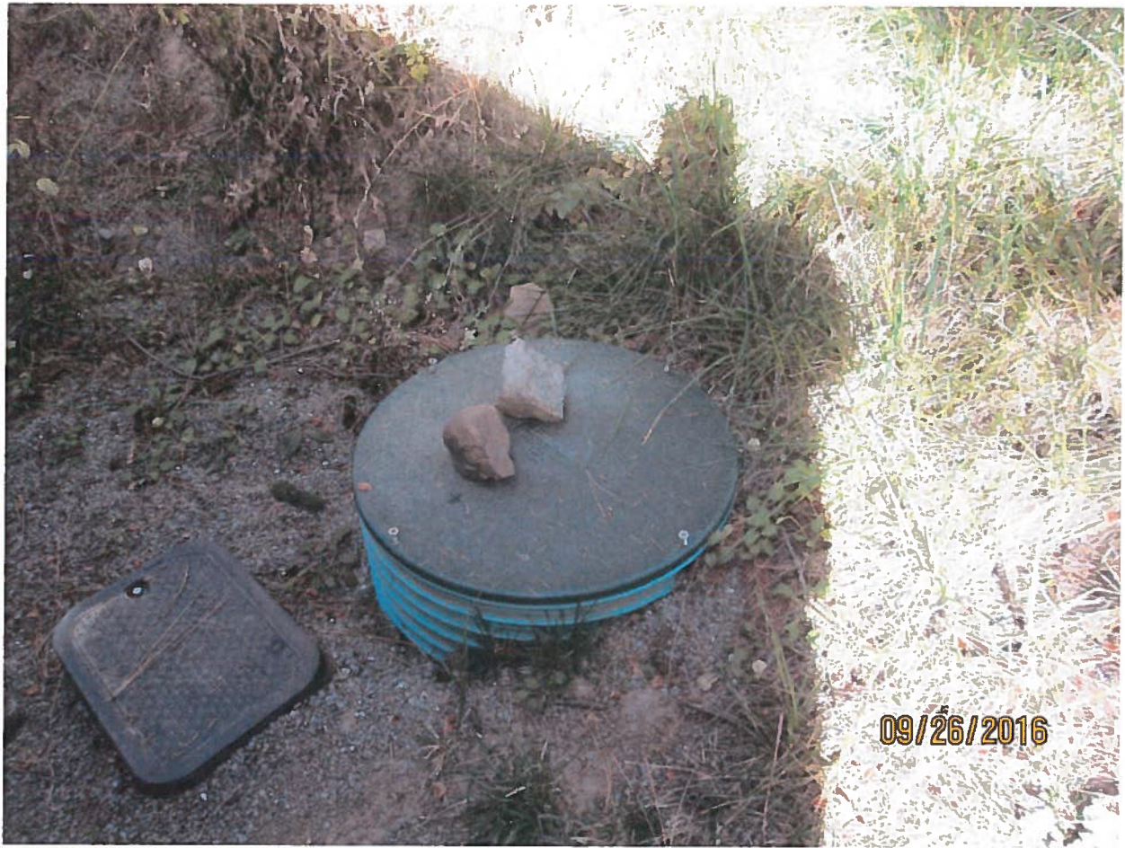
1,000 gallon cistern on system.
