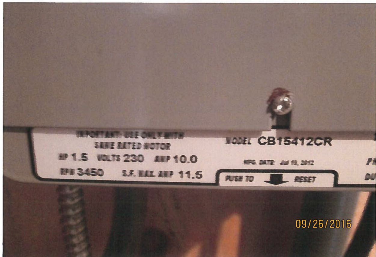
1.5hp pump in well.
