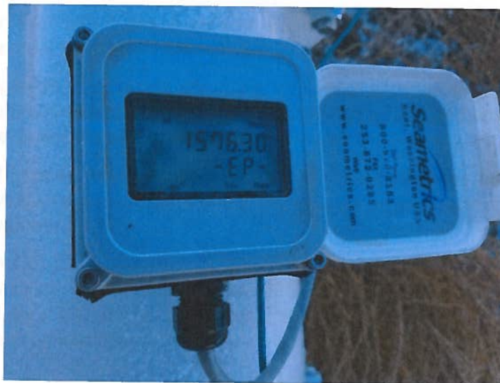
Figure 4. Well No. 1 flow meter – November 29, 2016 (totalized volume in acre feet)
