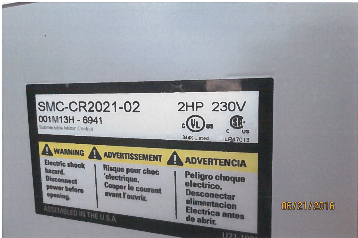
2hp submersible pump control box.
