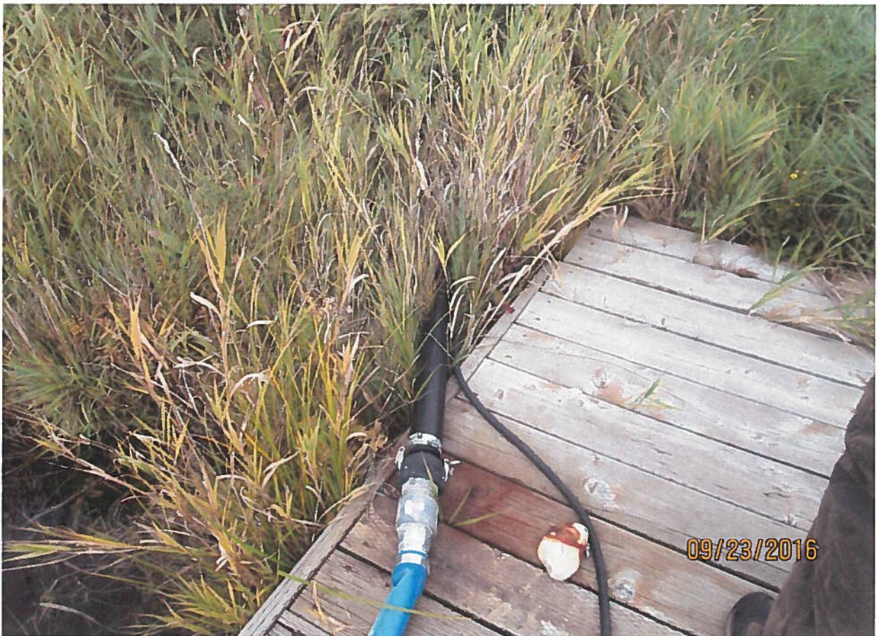
Piping going from pond to place of use. Pipe is buried from here.
