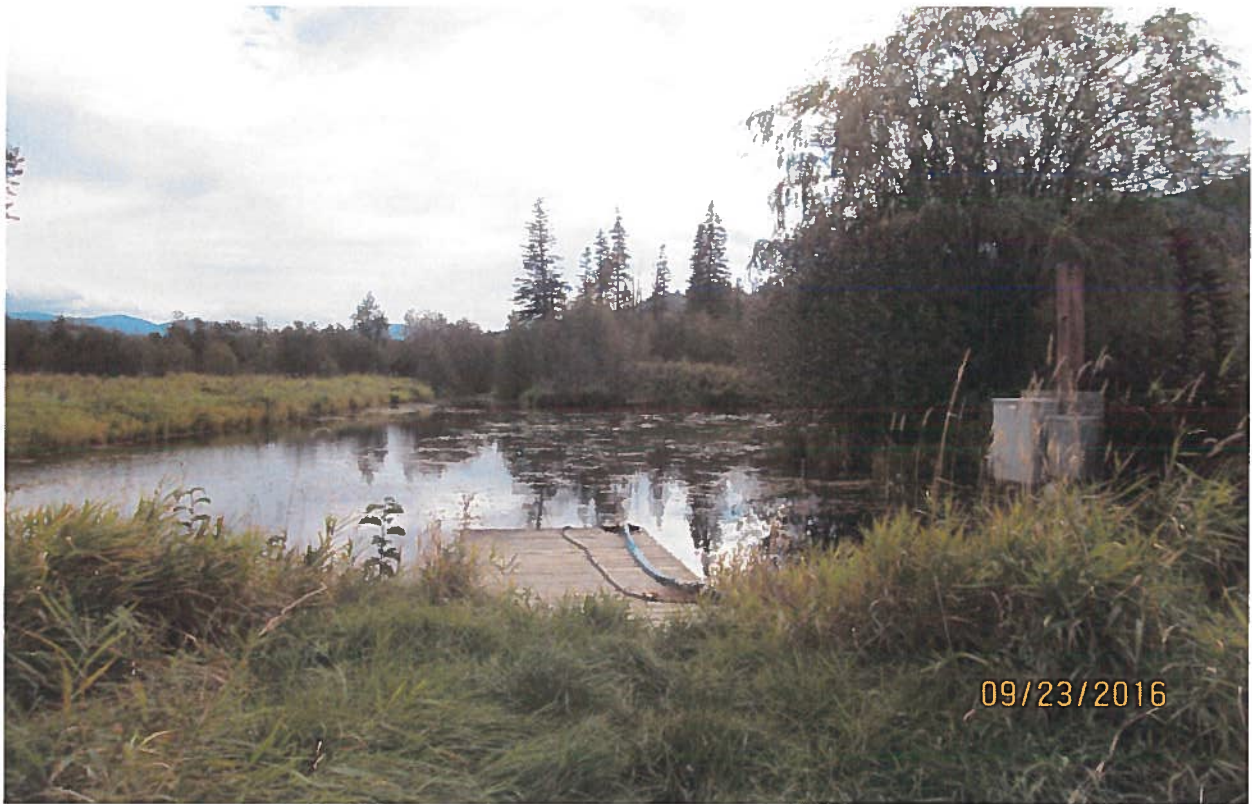
Overview of pond, dock, electrical box, and piping.
