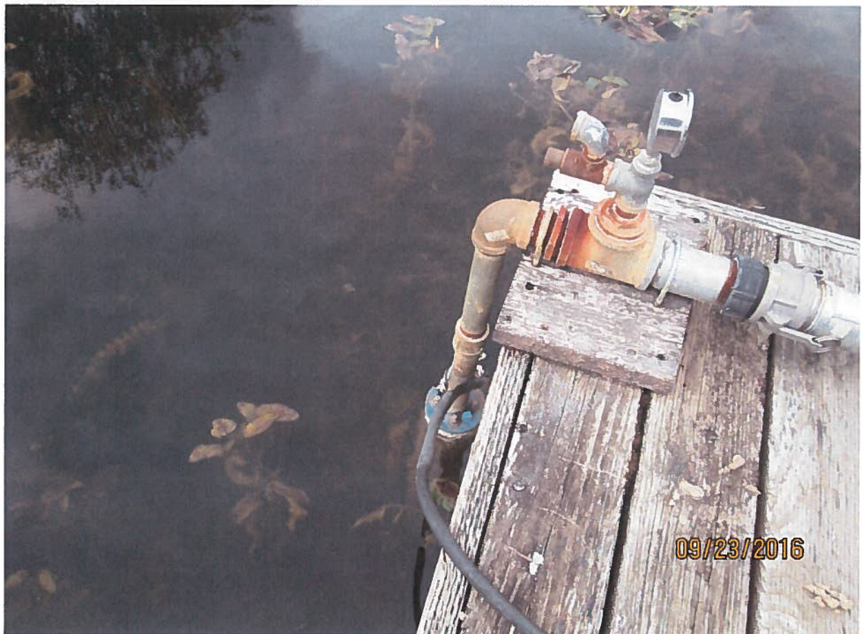
Diversion system from pond.
