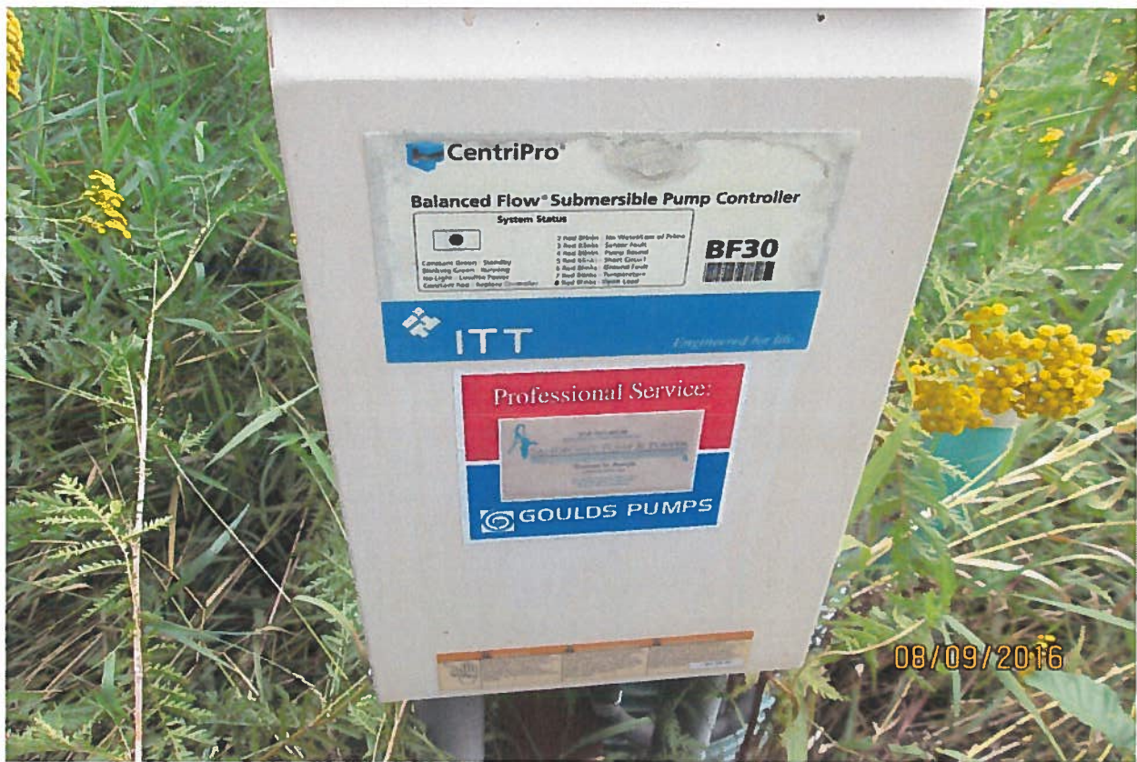
Control box on shore.
