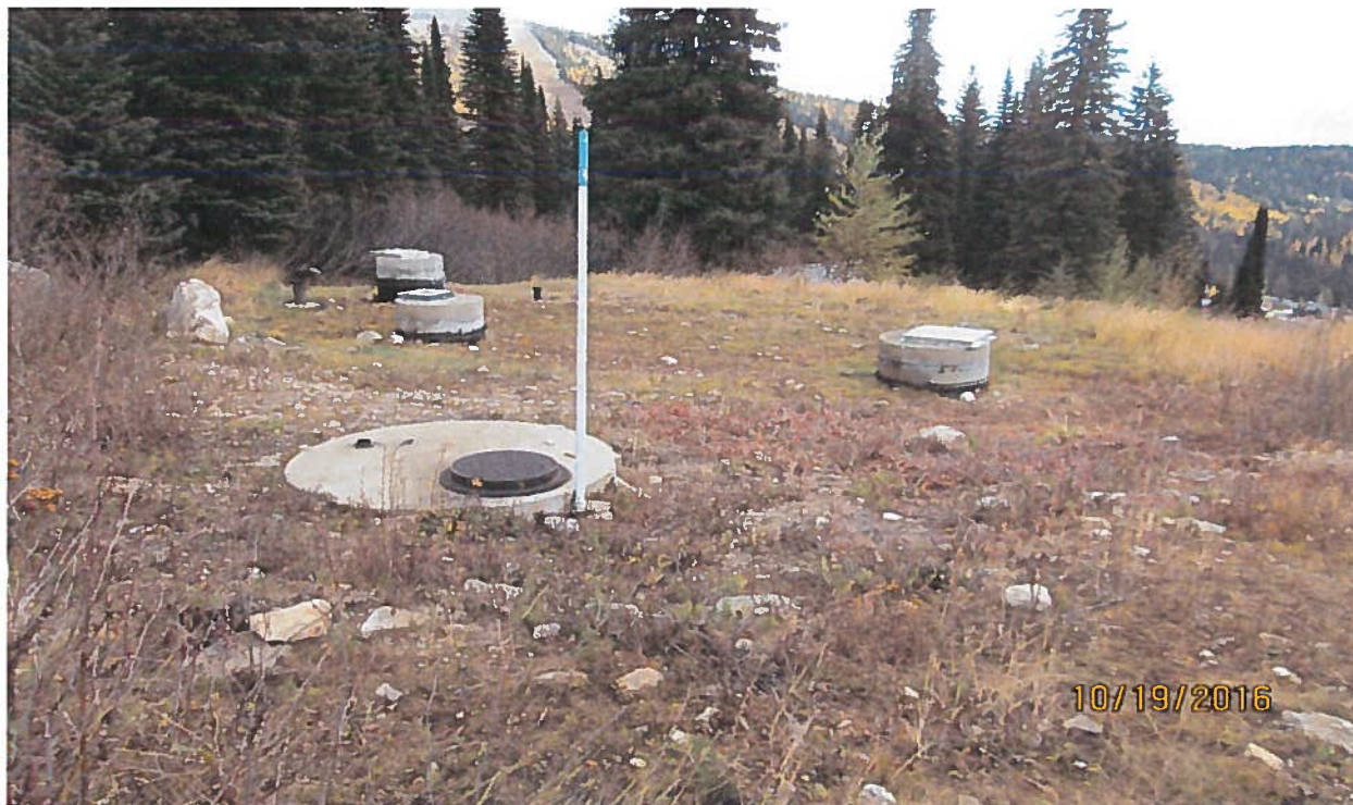
Reservoir next to where system pipes connect from wells and springs.
