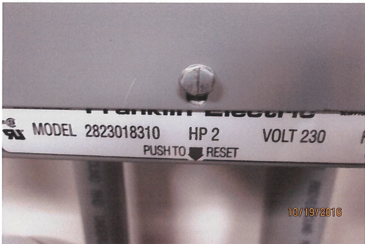
2 hp pump in well #6.
