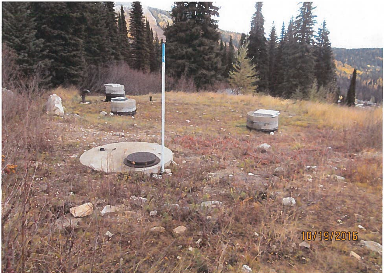
Top of 60,000 gallon reservoir.
