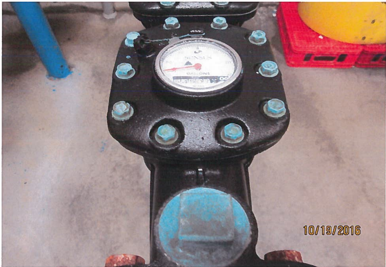
Flowmeter for well #5.
