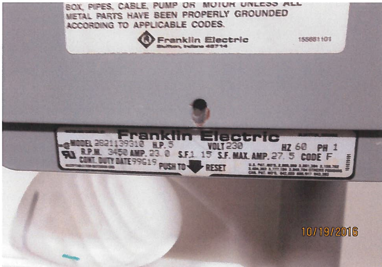
5 hp pump in well's #4 & #5.
