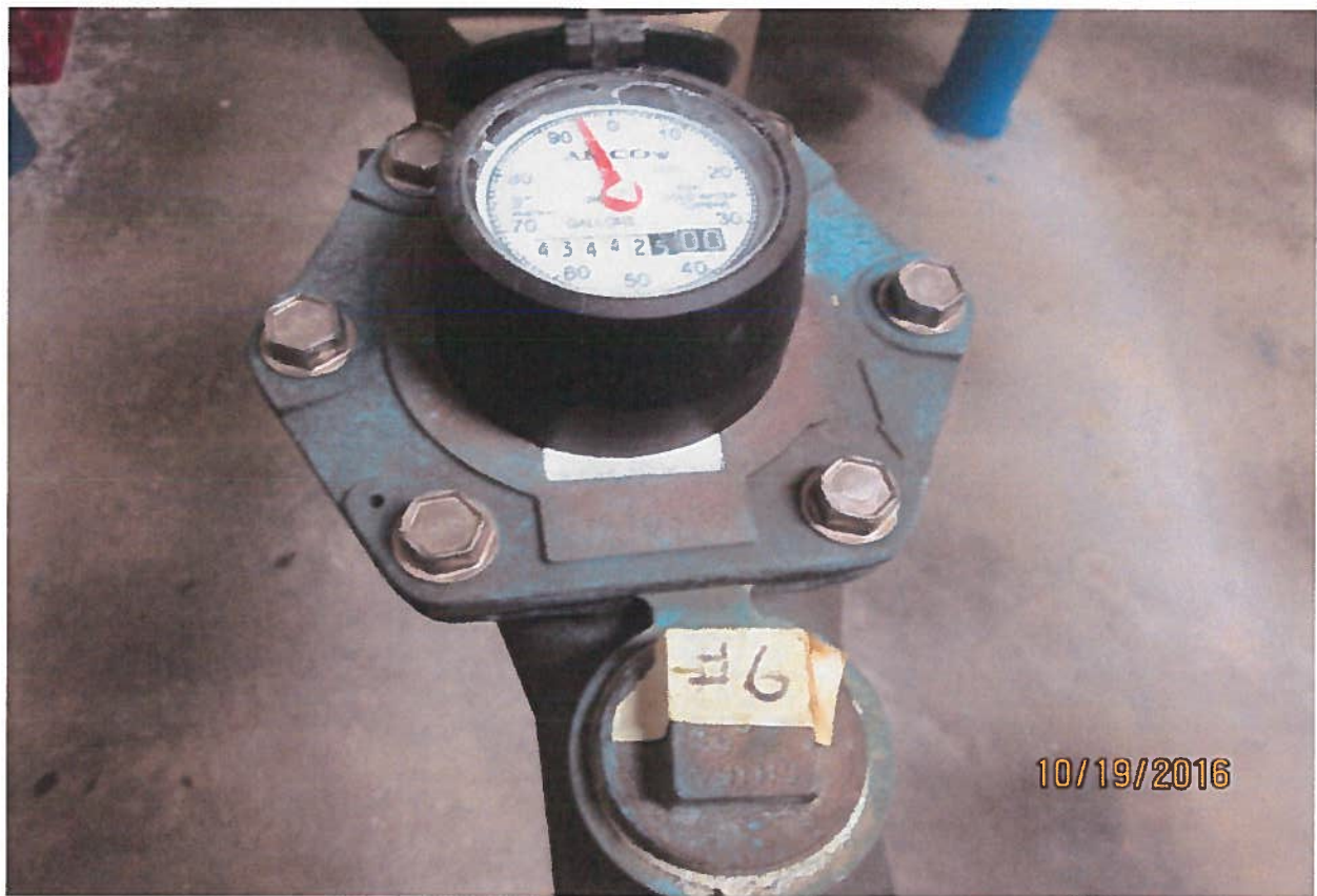
Flowmeter for well #6.
