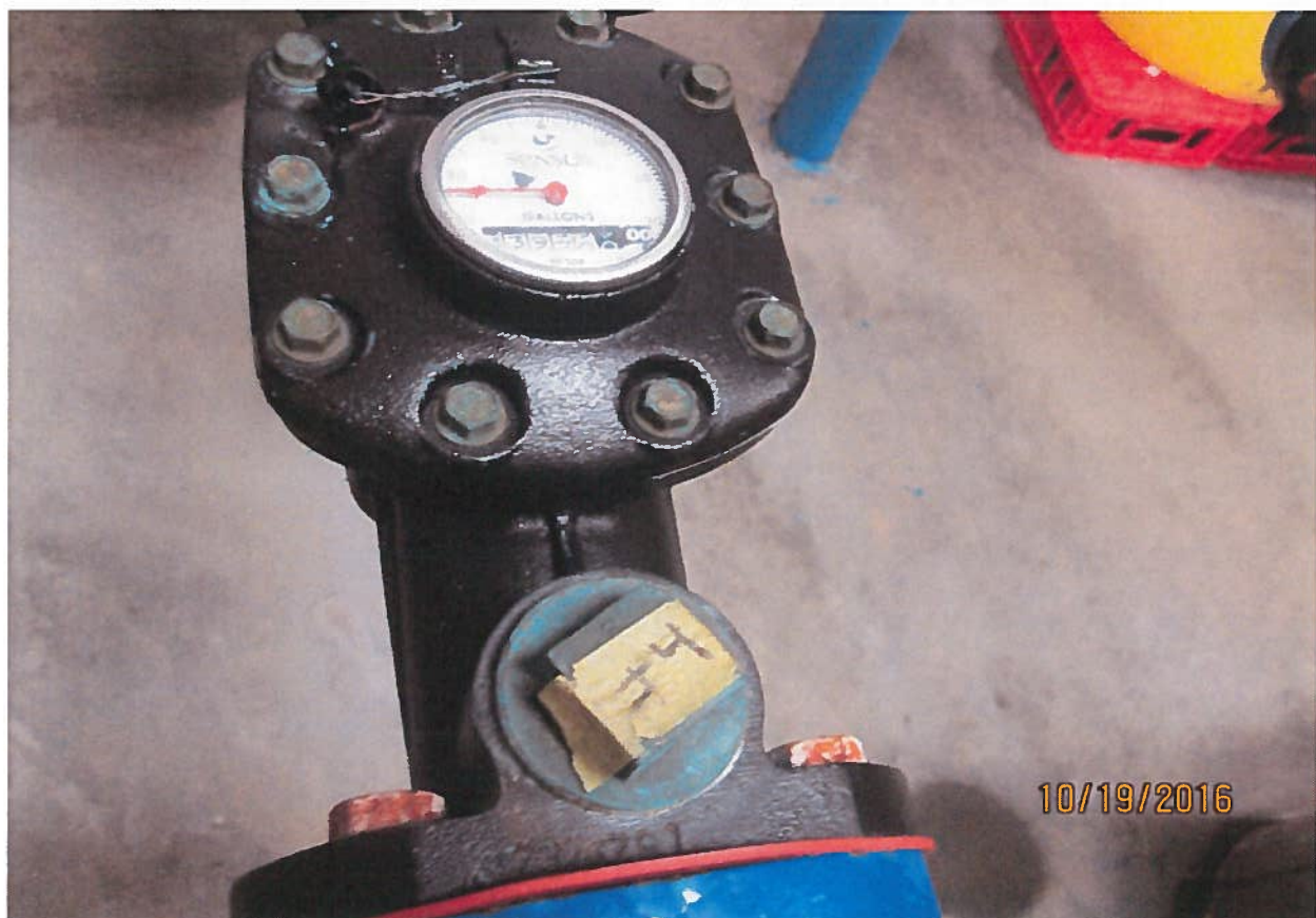
Flowmeter for well #4.
