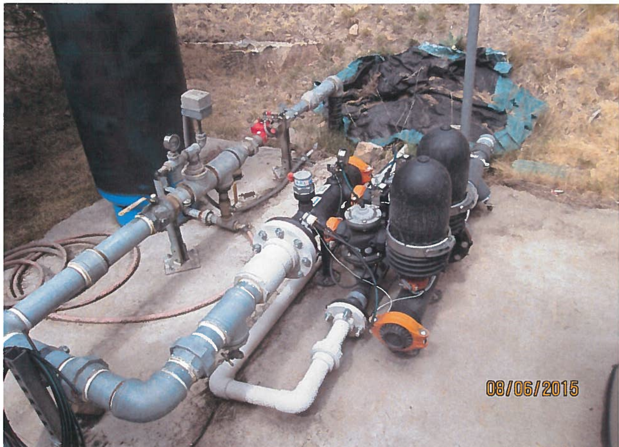
Filtration system for lake water. Water is pumped from lake to filtration to small storage tank and then pumped to irrigation system.
