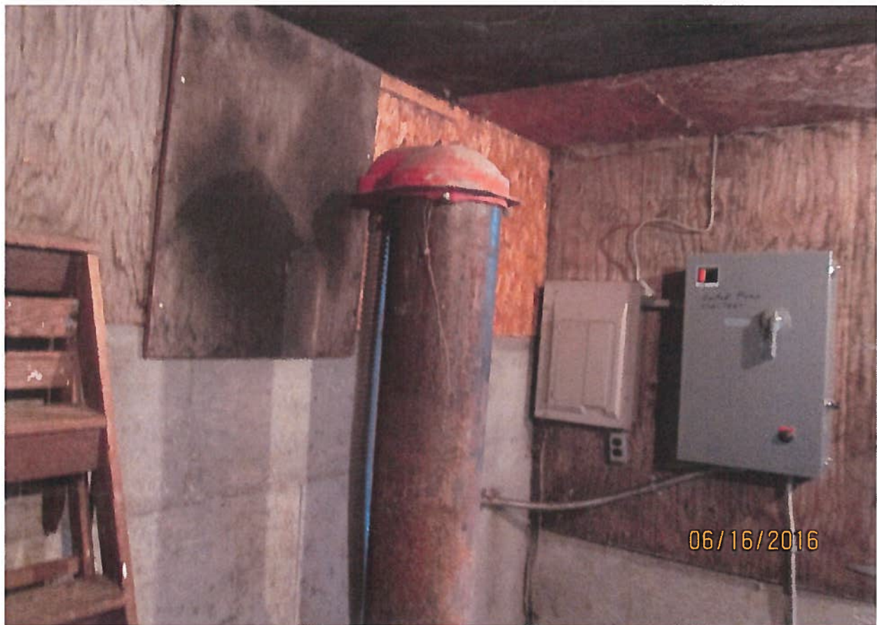
Well with 10hp pump running at 60 psi. Given IDWR tag A0015438.
