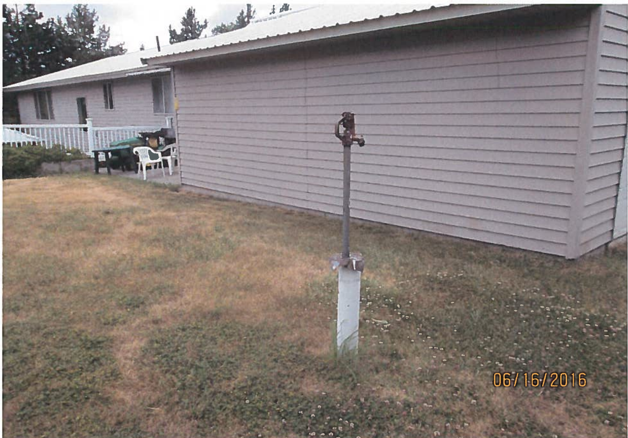
Frost free hydrant for irrigation.
