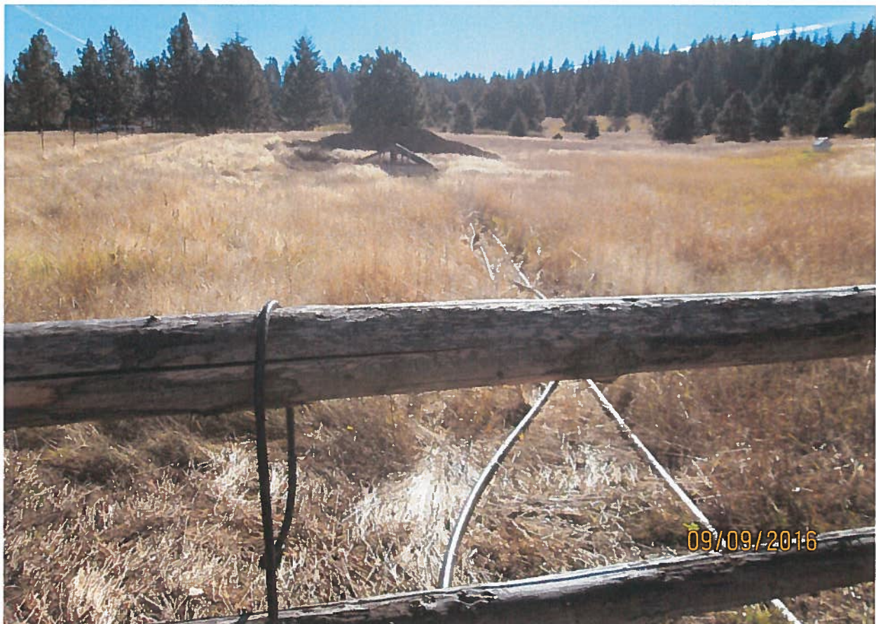
Storage tank with hoses from portable pump. In upper right you can see spring house.
