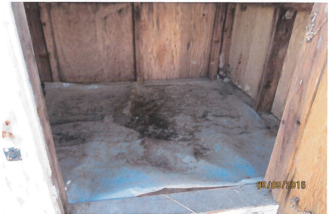
Inside spring house. Spring box was covered to protect water.
