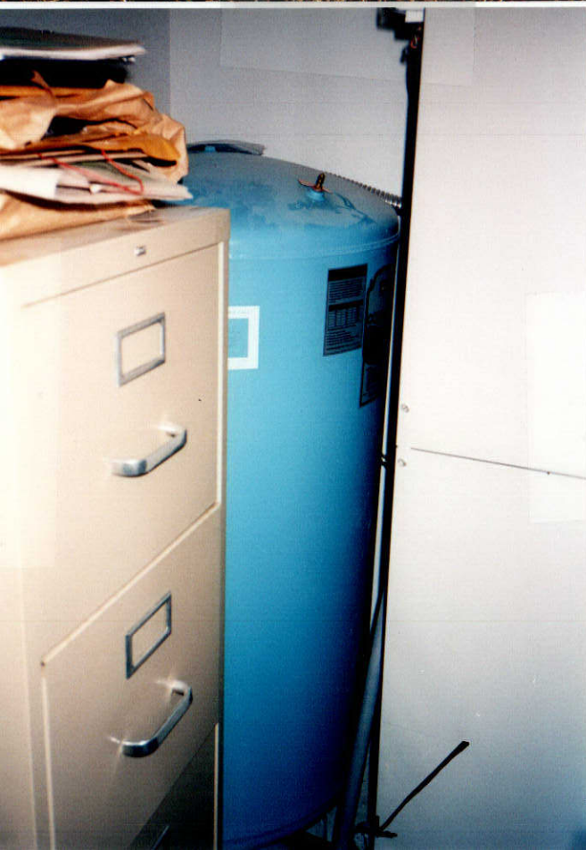
← 2. Pressure tank in home.
