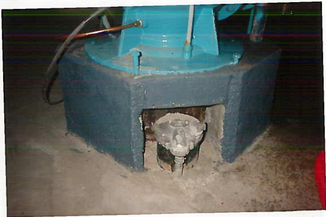
PHOTO TWO- Well inside of well house. Boise Water Corp. constructed their well, 16" casing, next to church well.
