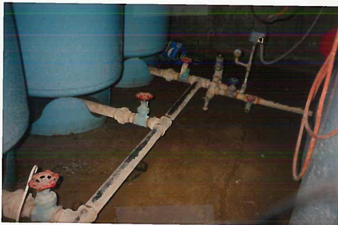
PHOTO FOUR- Pressure tanks in underground concrete vault.
