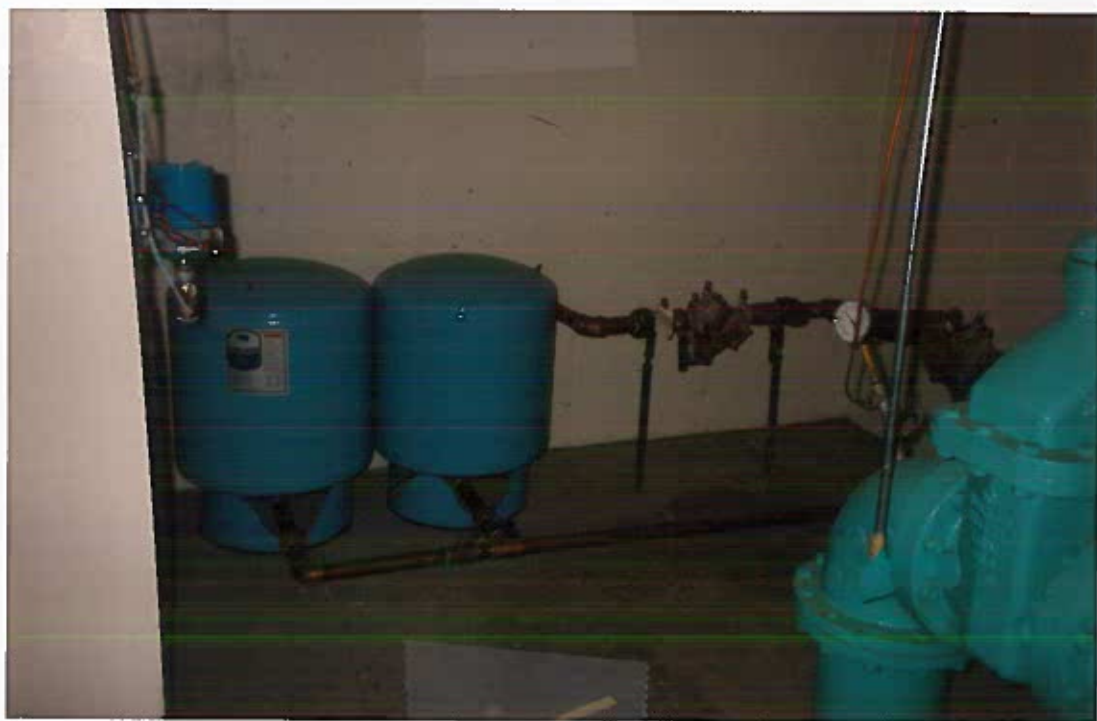
PHOTO THREE- Two of six Pressure Tanks in well house.
