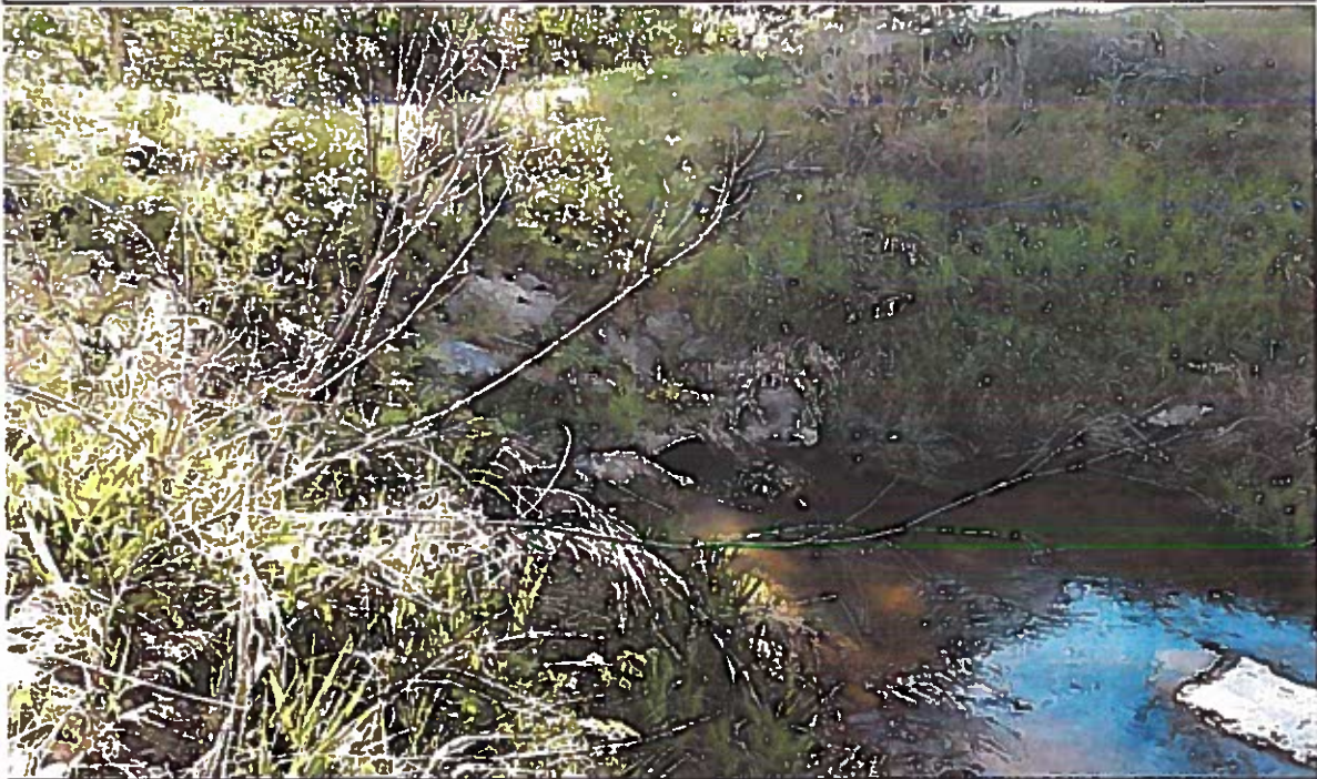
View southeasterly of the 36" CMP discharge pipe from the Boise River to the headwaters of Warm Springs Creek.
