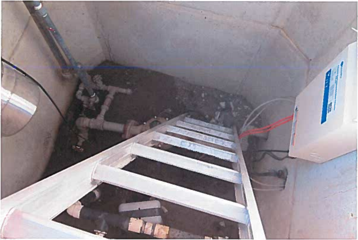
Pump station at Trumpeter Well
