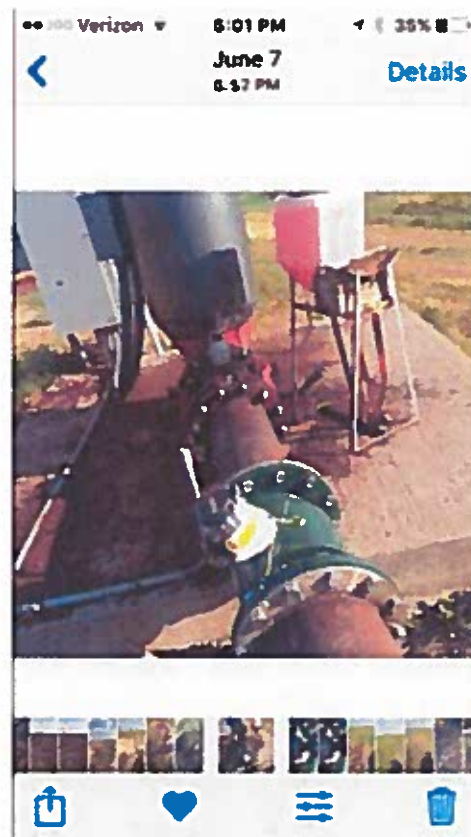
Pump, Well, and Flow Meter
