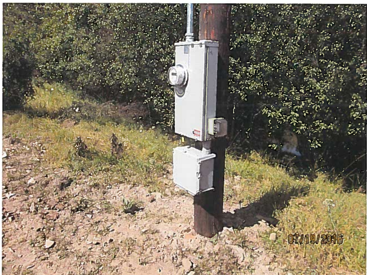
Point of diversion on Benewah Creek. Pump was getting repaired at time of exam.
