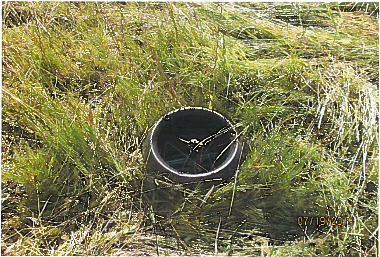
Sprinkler head off of Benewah Creek.
