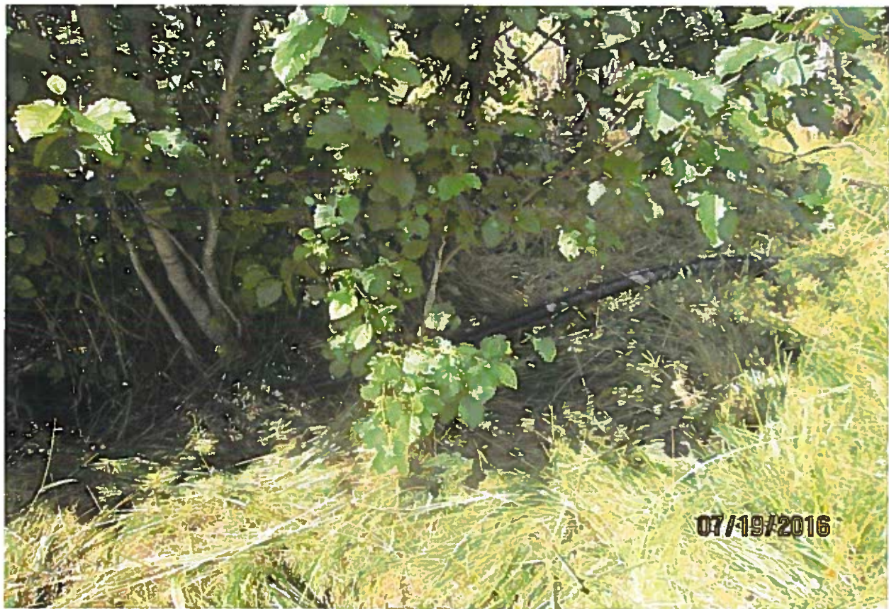
PVC piping heading to sprinklers from point of diversion.
