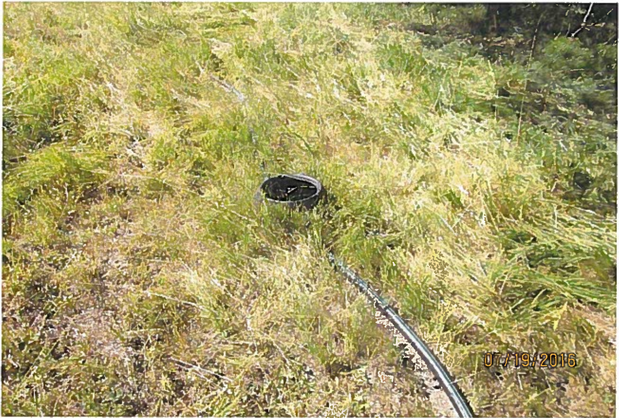
1 line of sprinklers located in Lot 3.
