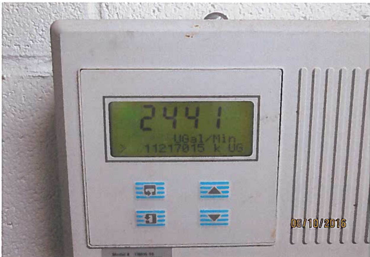
Pump 3 signal converter. 2,450gpm was reached after photo was taken.
