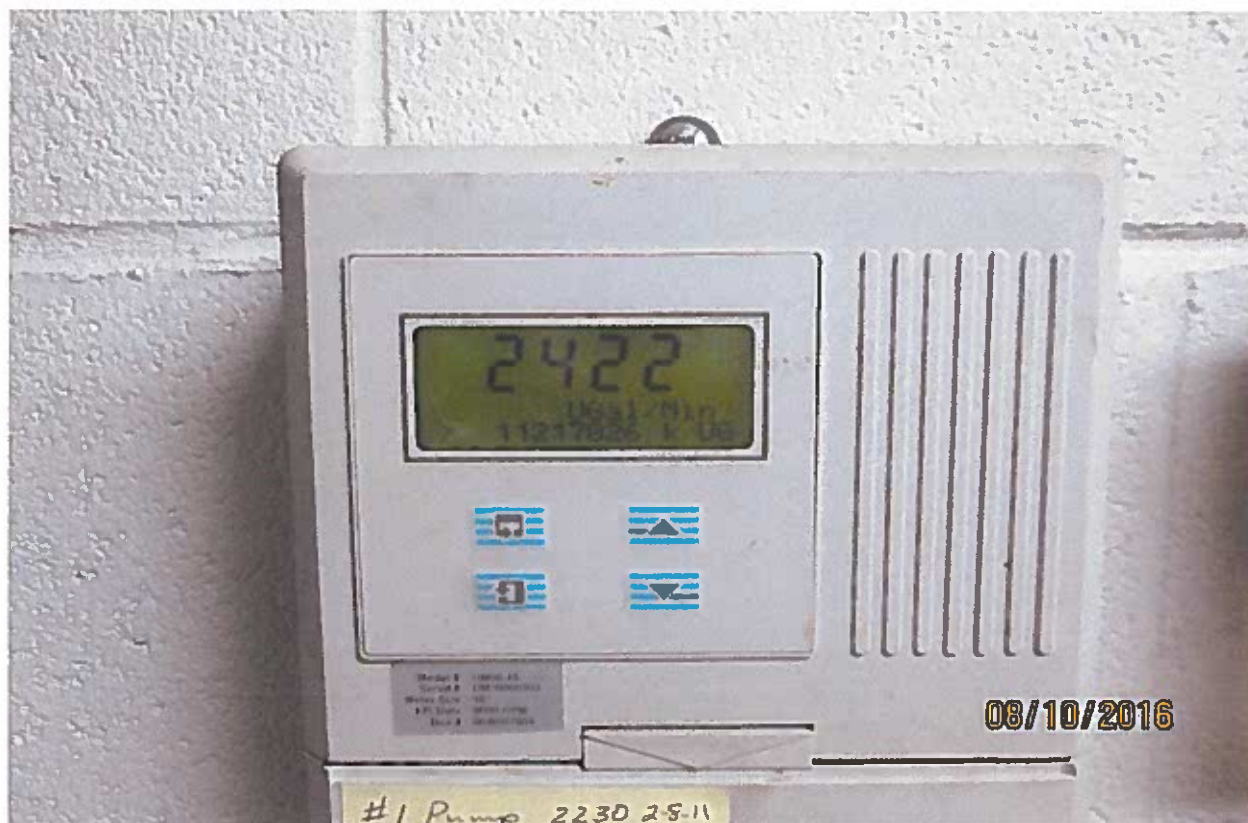
Pump 2 signal converter.
