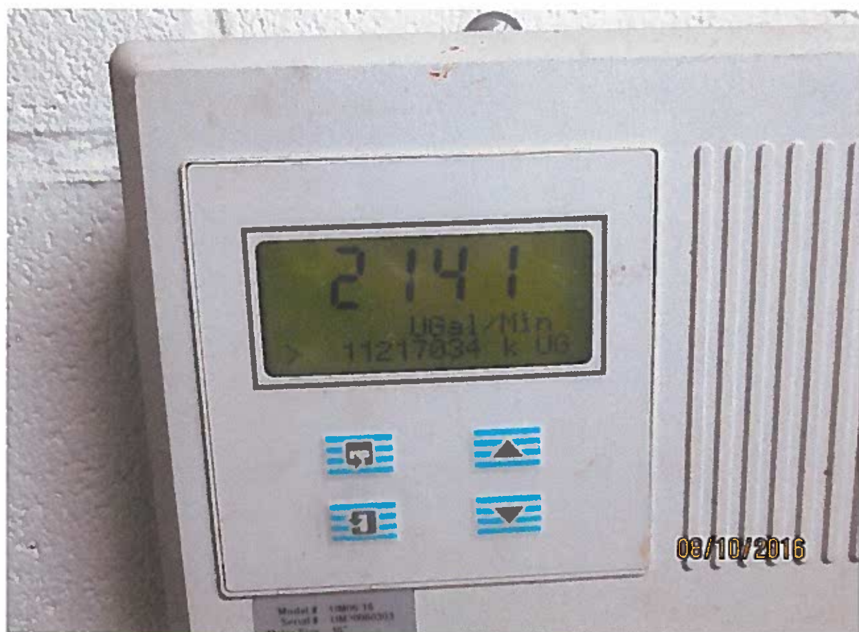
Pump 1 signal converter.
