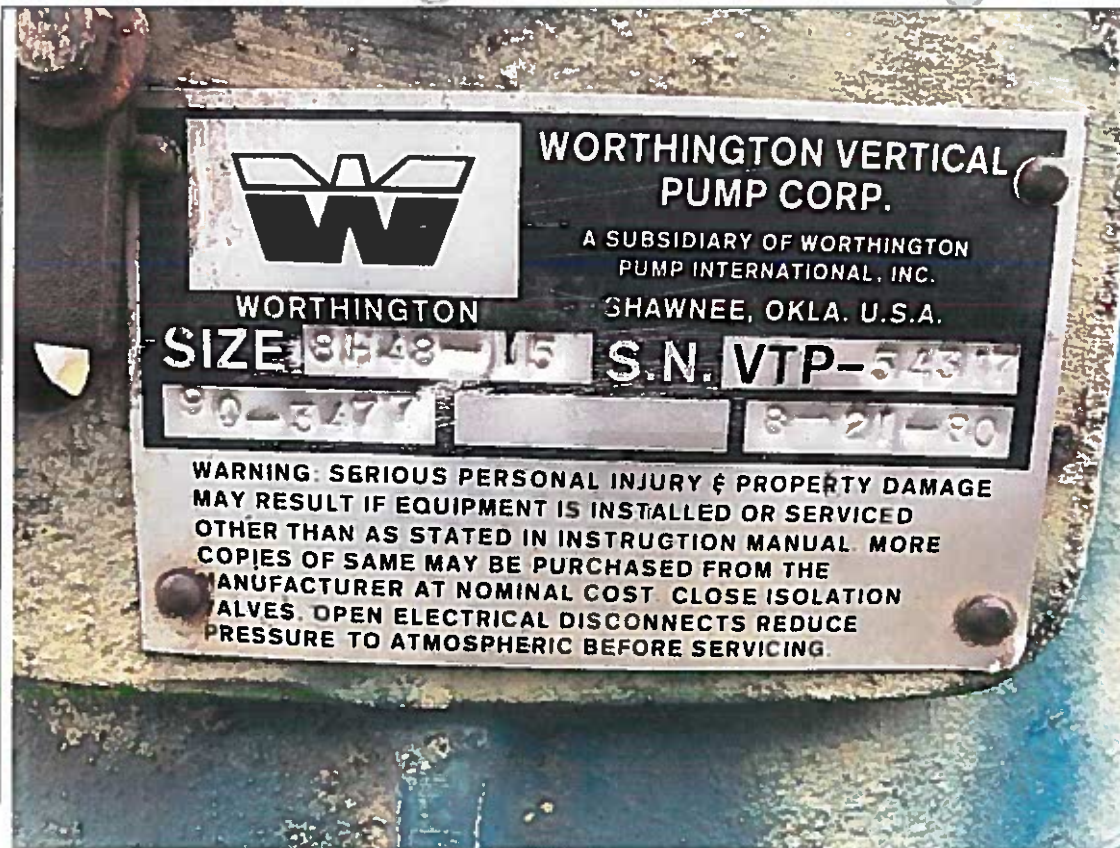
Worthington Vertical Pump Corp tag
