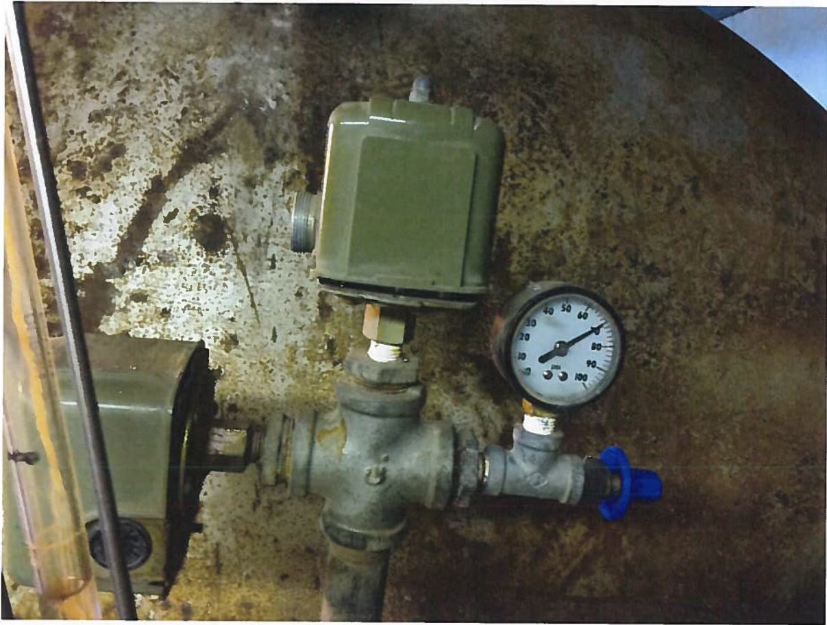
10. Pressure gage. Normal discharge pressure is 70 psi.
