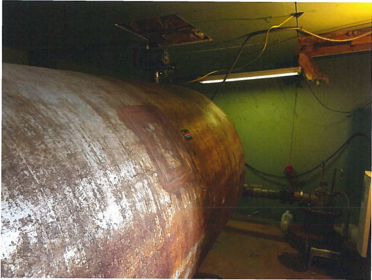
4. Nominal 1500-gallon hydropneumatics tank (left) and well head (right).
