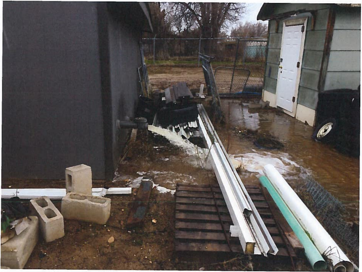
2. Flush to waste during flow test at back of well house.
