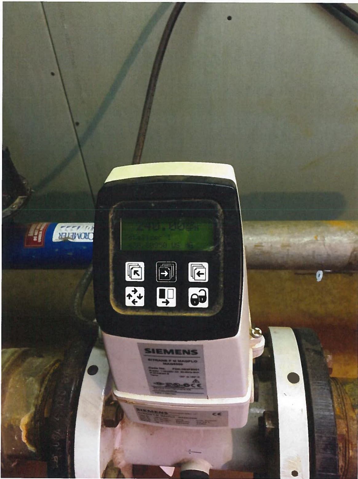
11. Flow meter reading (240 gpm) during 10-minute flow test.
