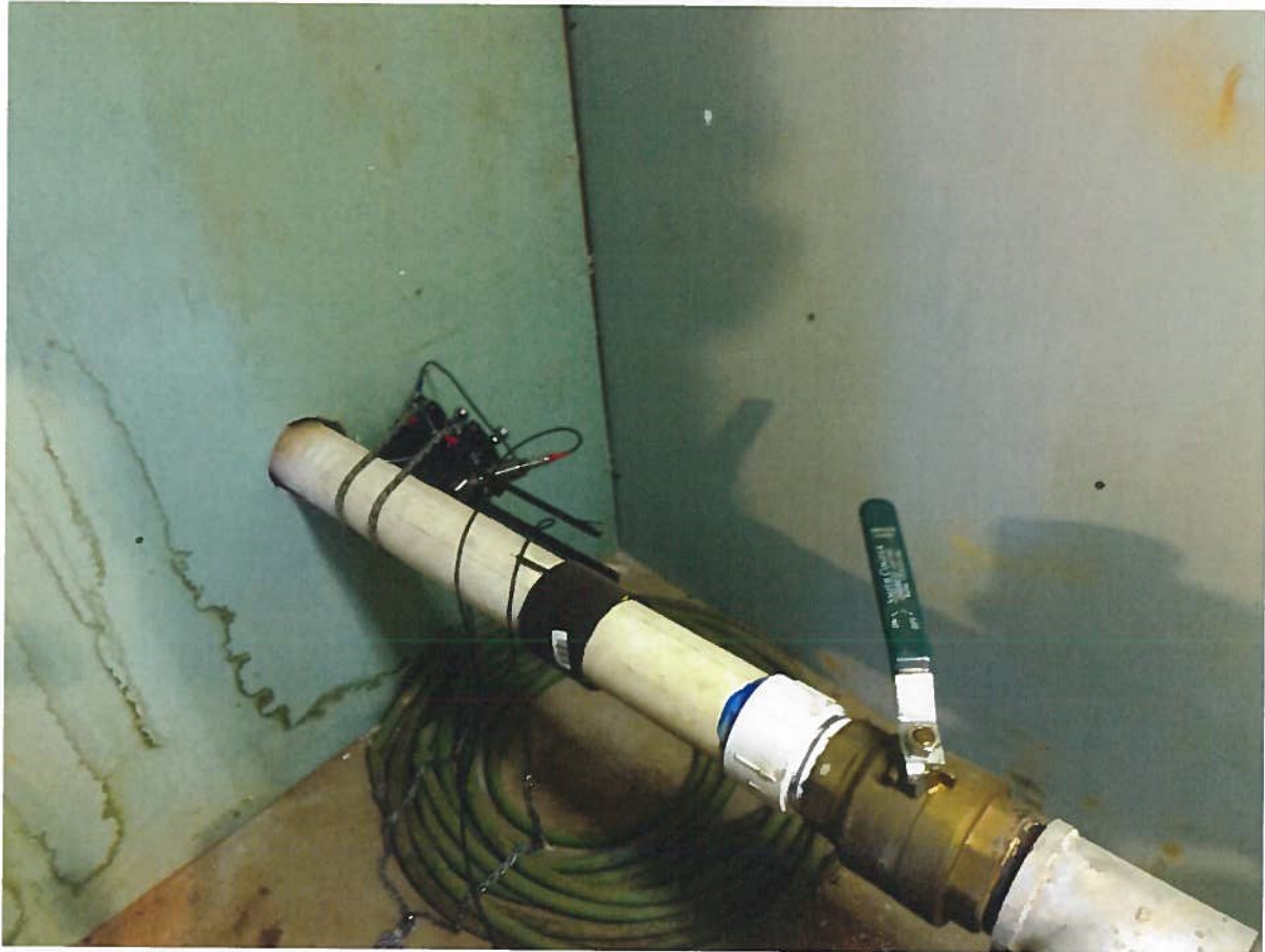
12. Location for portable ultrasonic flow meter on flush-to-waste pipe during flow test. Turbulence downstream of ball valve was too great to allow for reading.
