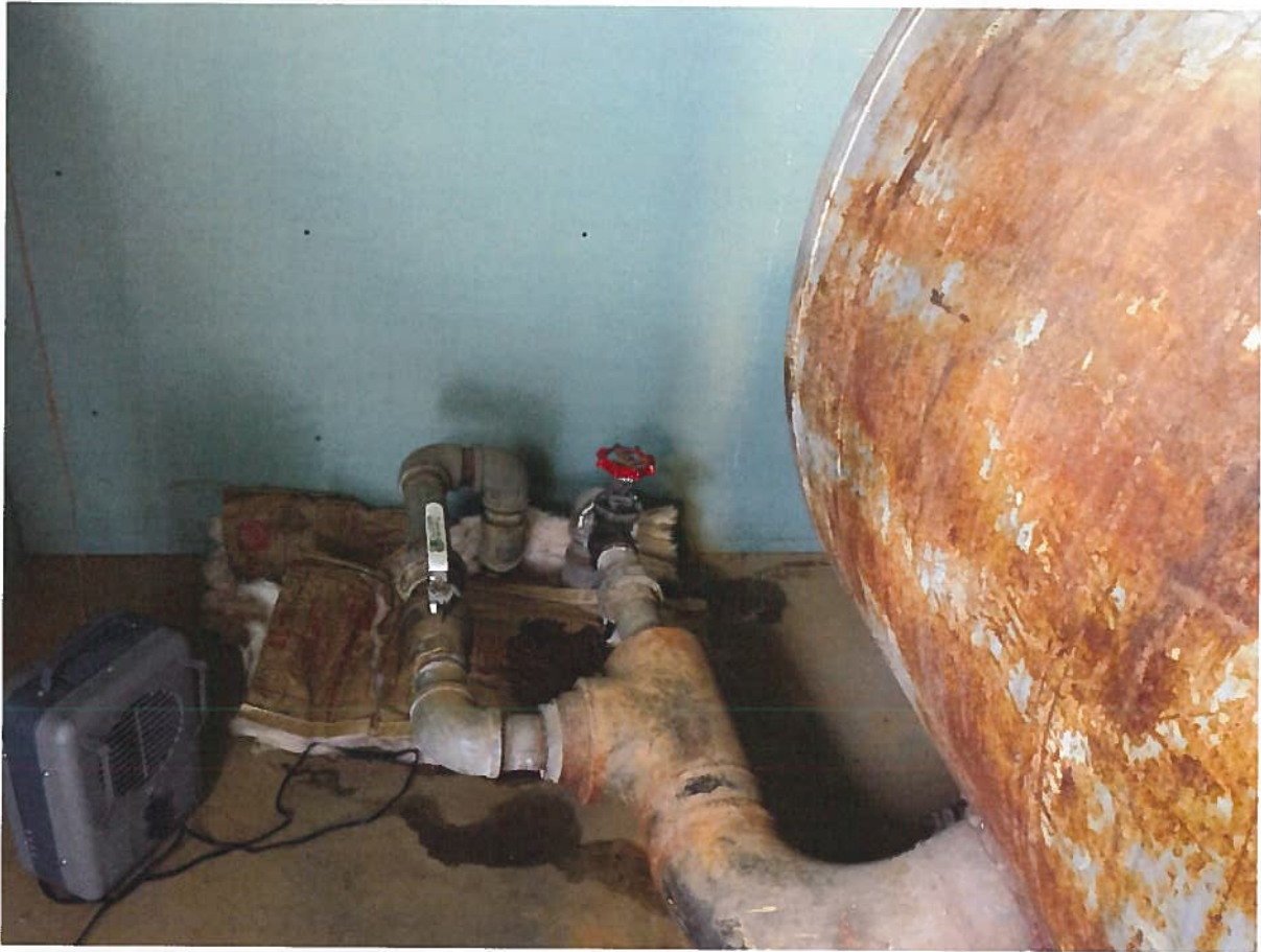
5. Discharge piping from hydropneumatics tank to water system.
