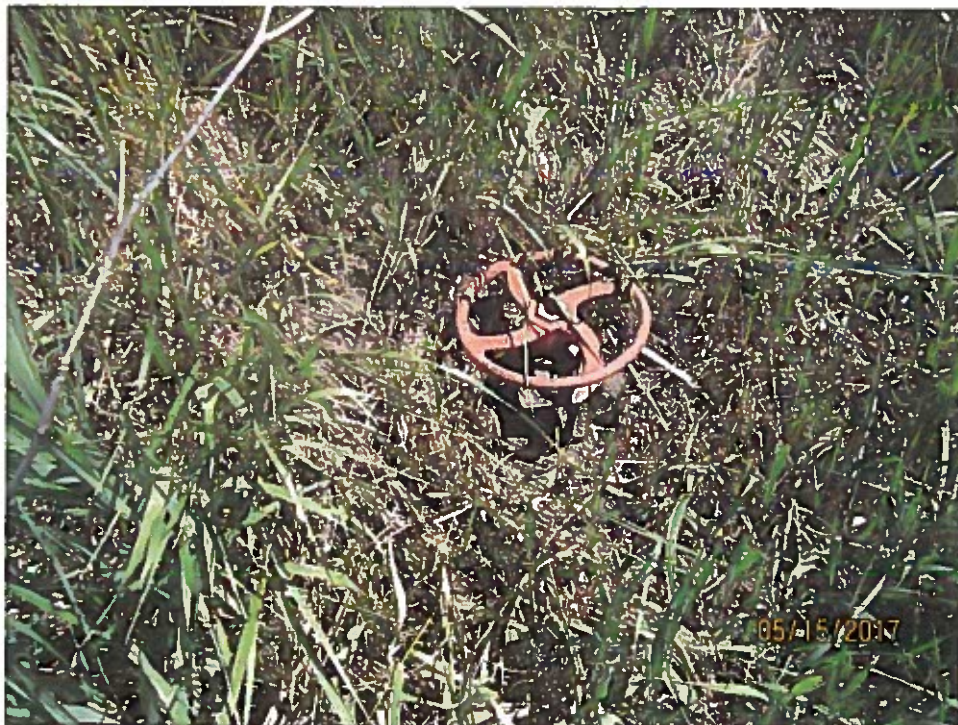
Figure 4 The valve used to release water from the pond.
