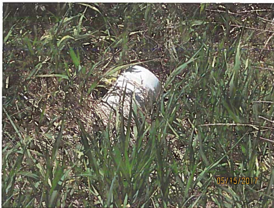
Figure 5 The 6" PVC pipe coming out from under the dam. The water is release from the dam and conveyed along the excavated ditch to the irrigation place of use.
