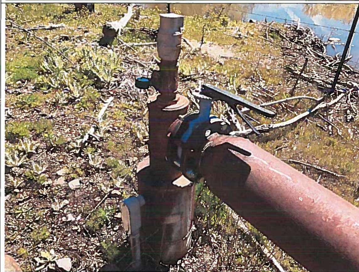
10" well discharges to pipe shown on right.
