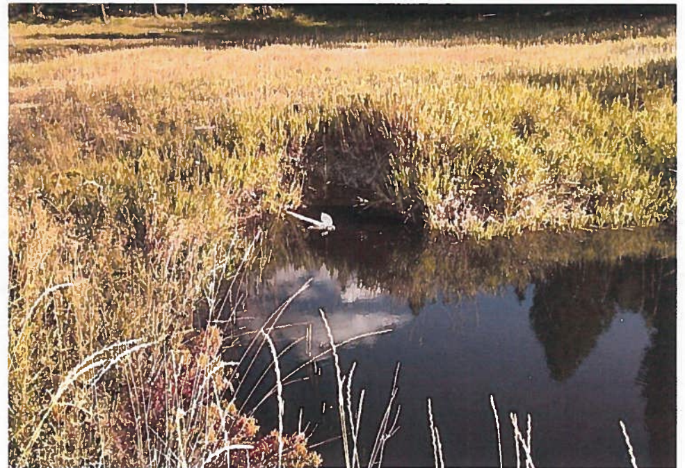
87-10071 LONG CREEK BACKGROUND - FILL PIPE TO POND
