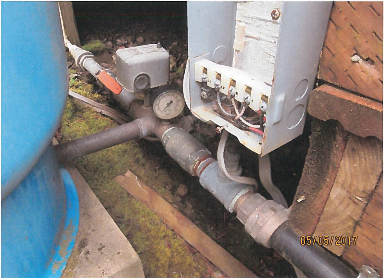
Pump box next to pressure tank. 1/2hp pump was broken at time of exam.
