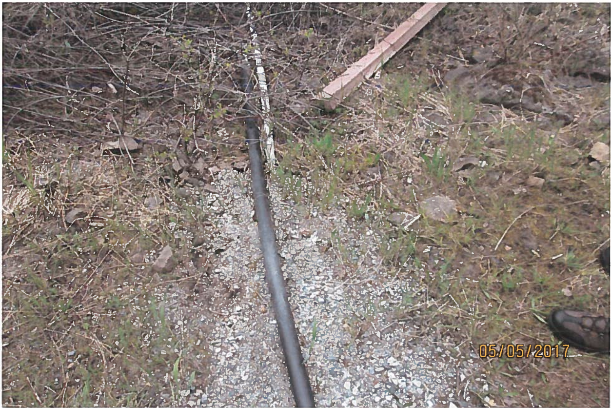
Water line on shore.
