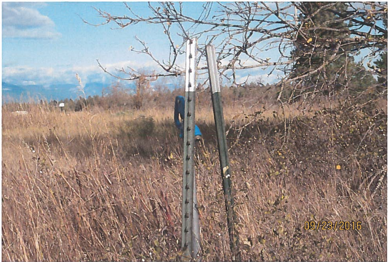
Frost free hydrant for stub in for home 3. 5 gallon bucket test performed here.
