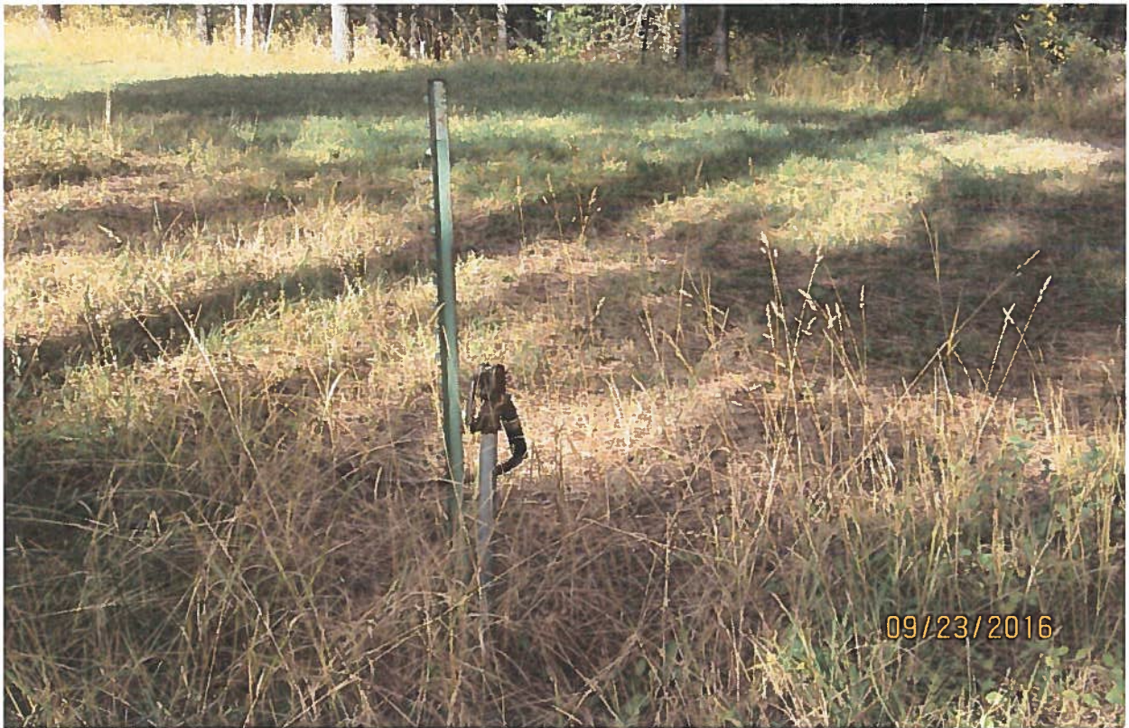
Frost free hydrant used for irrigation.
