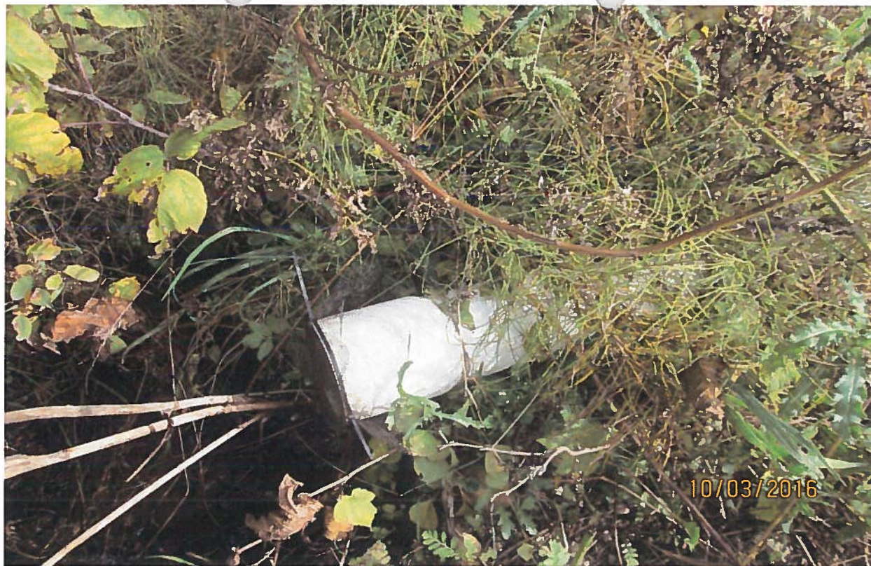
End of overflow pipe back into unnamed stream.
