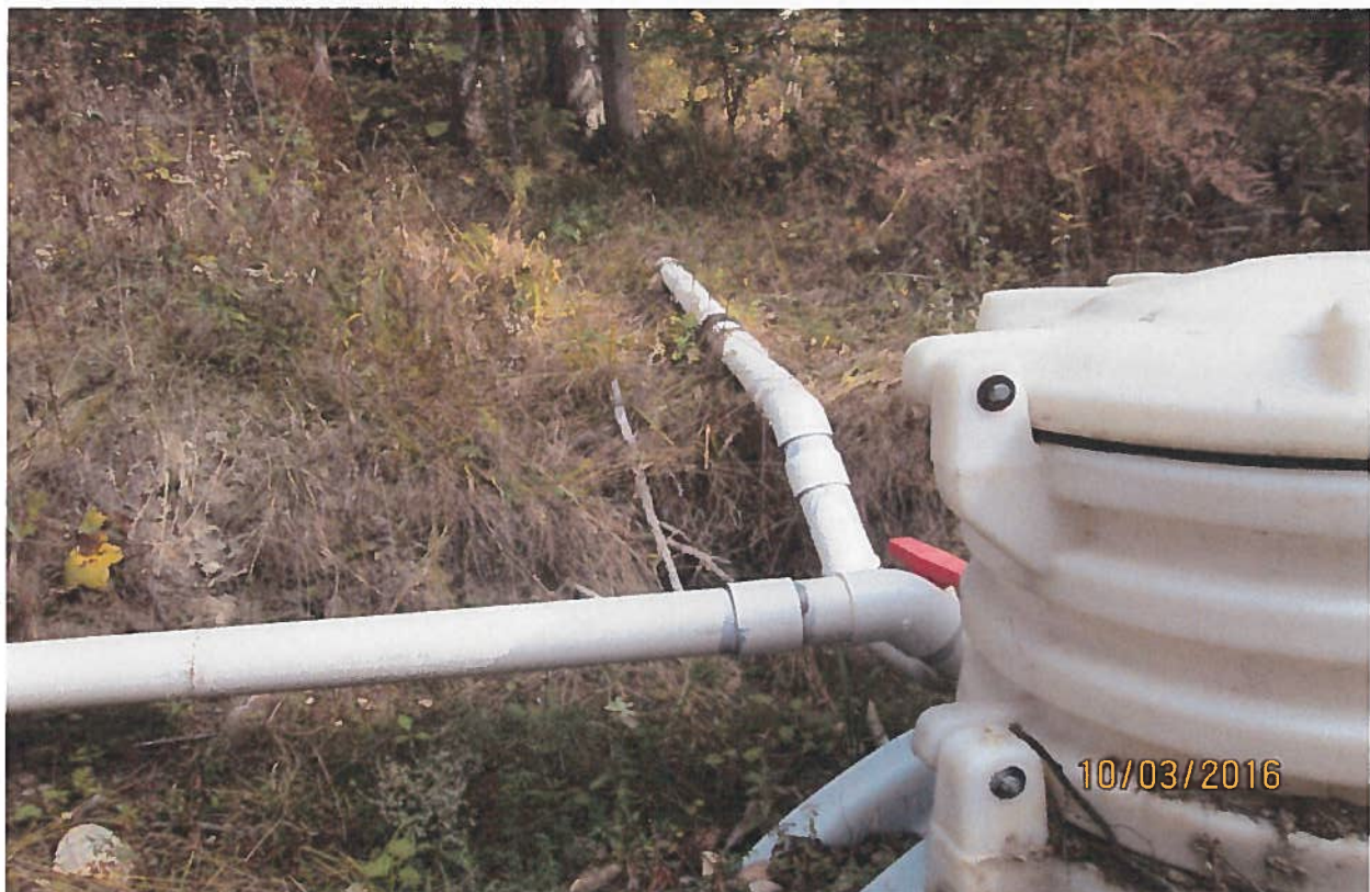
Looking up towards point of diversion. 4 inch pipe fed into 1,800 gallon cistern. Pipe going to left is overflow back into unnamed stream.
