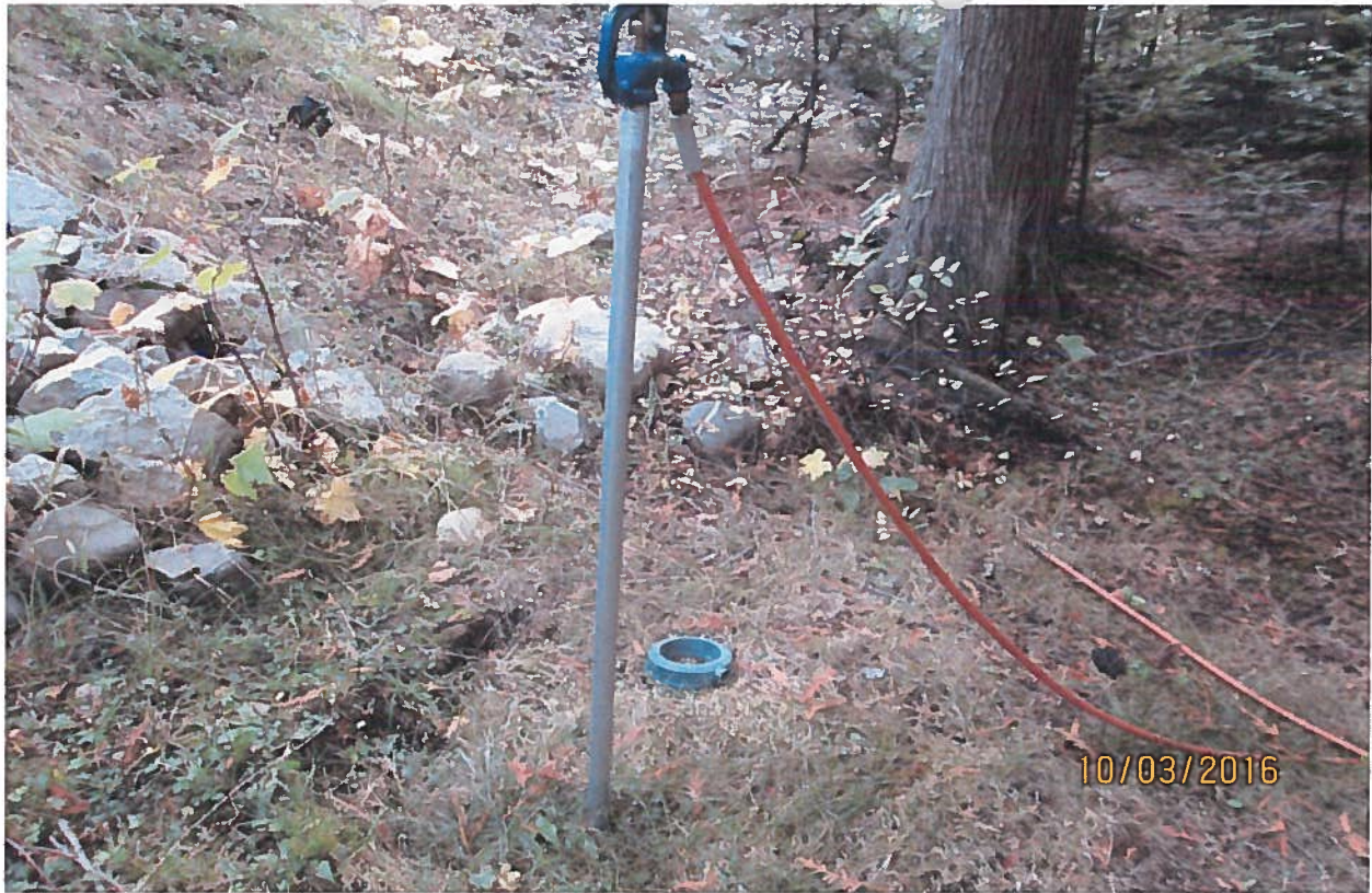
Frost free with hose and irrigation of yard.
