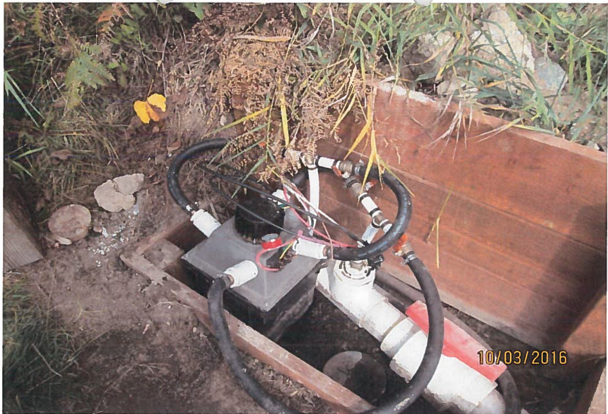
Hydropower unit with four 3/8 heads. Applicant only uses two heads at a time. Put in extra two units in case one or two heads get broke or stop working he can switch to other heads to keep power going.
