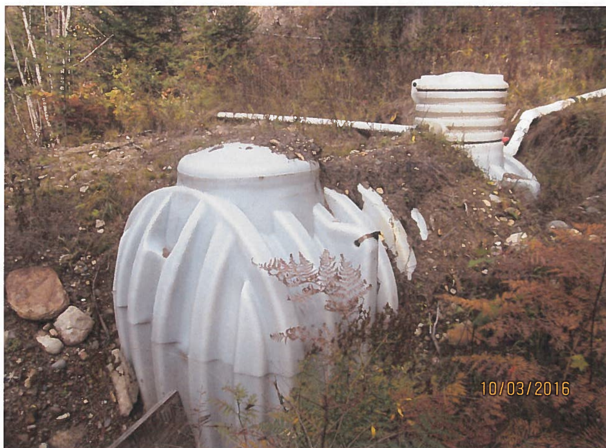
Cistern with inflow pipe and overflow pipe.
