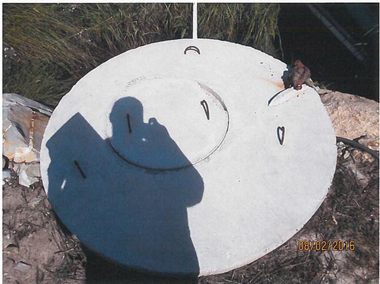
Mirror Creek point of diversion. 1/2hp pump in culvert.
