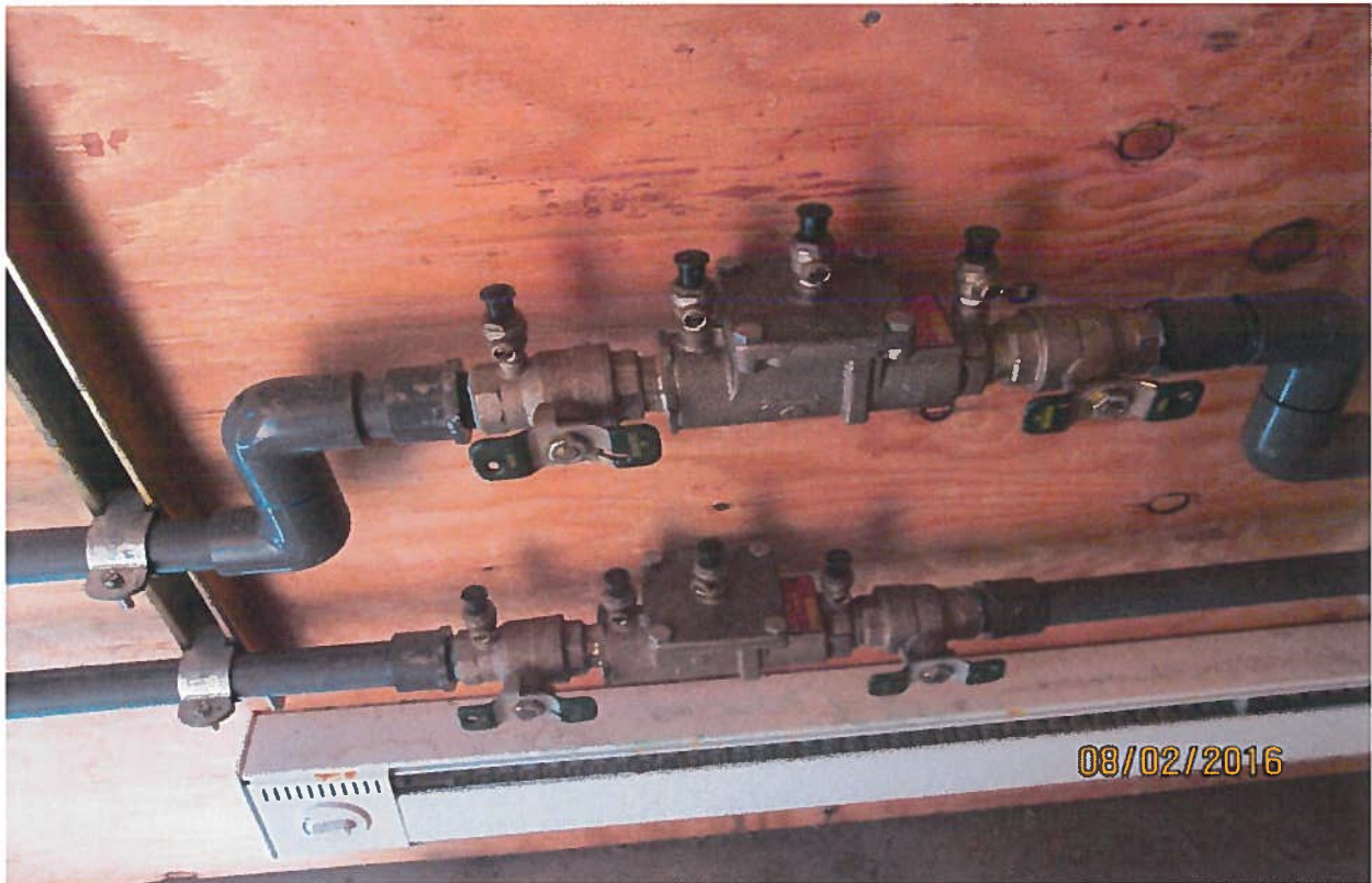
Backflow preventers on each source prior to pipes combining into one.
