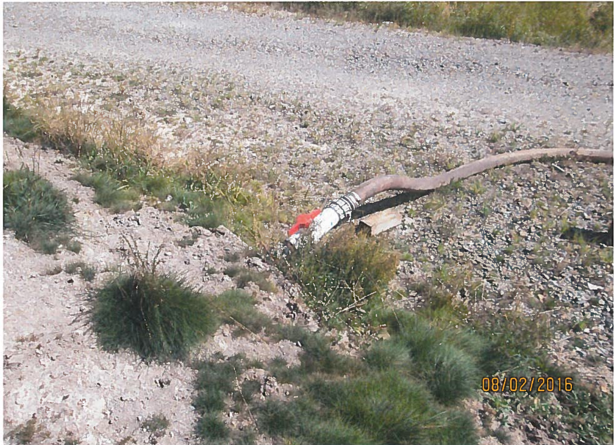
Outlet pipe on outside of dam with check valve.
