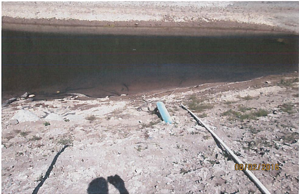
Outlet pipe for irrigation.
