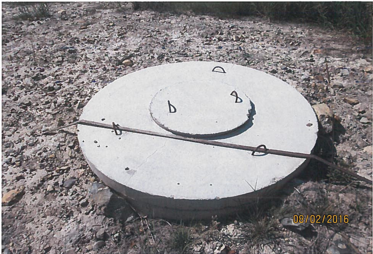
Hand dug cistern well. 1/2hp pump in well.
