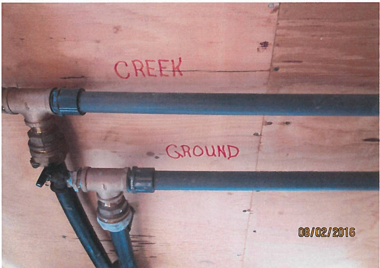
Water pipes from each source inside pump house.
