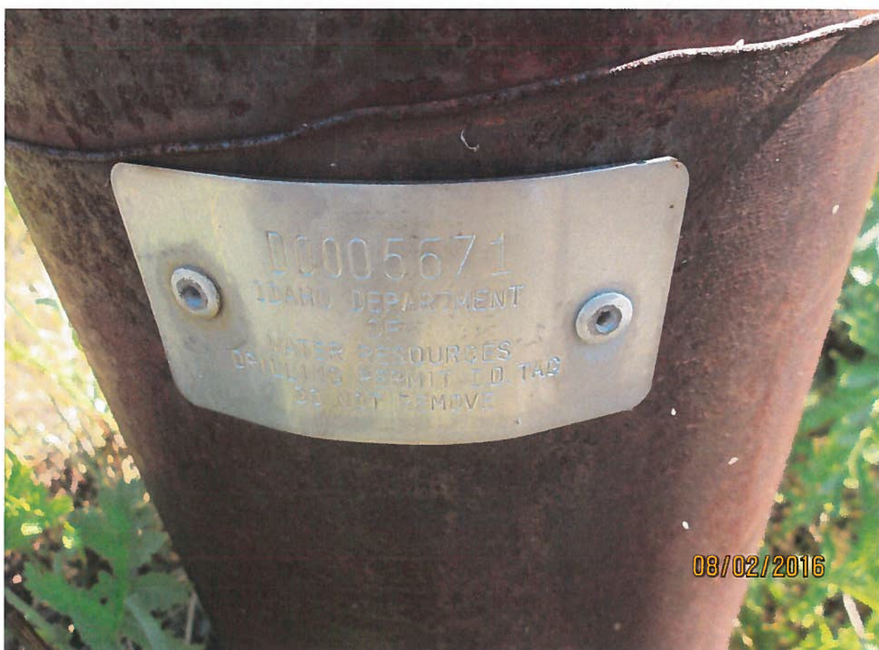
Well D0005671 given IDWR tag A002004. 7.5hp pump in well that produced 100 gpm per flow meter.
