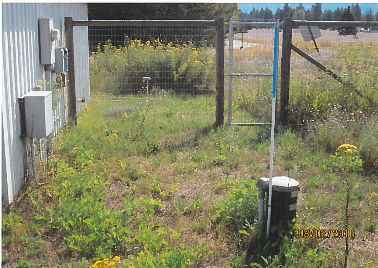
Location of both wells adjacent to pump house.
