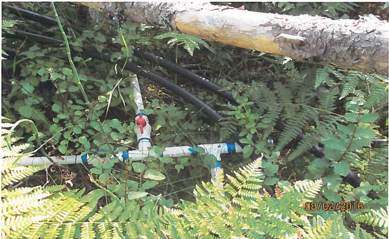
PVC piping running around property.
