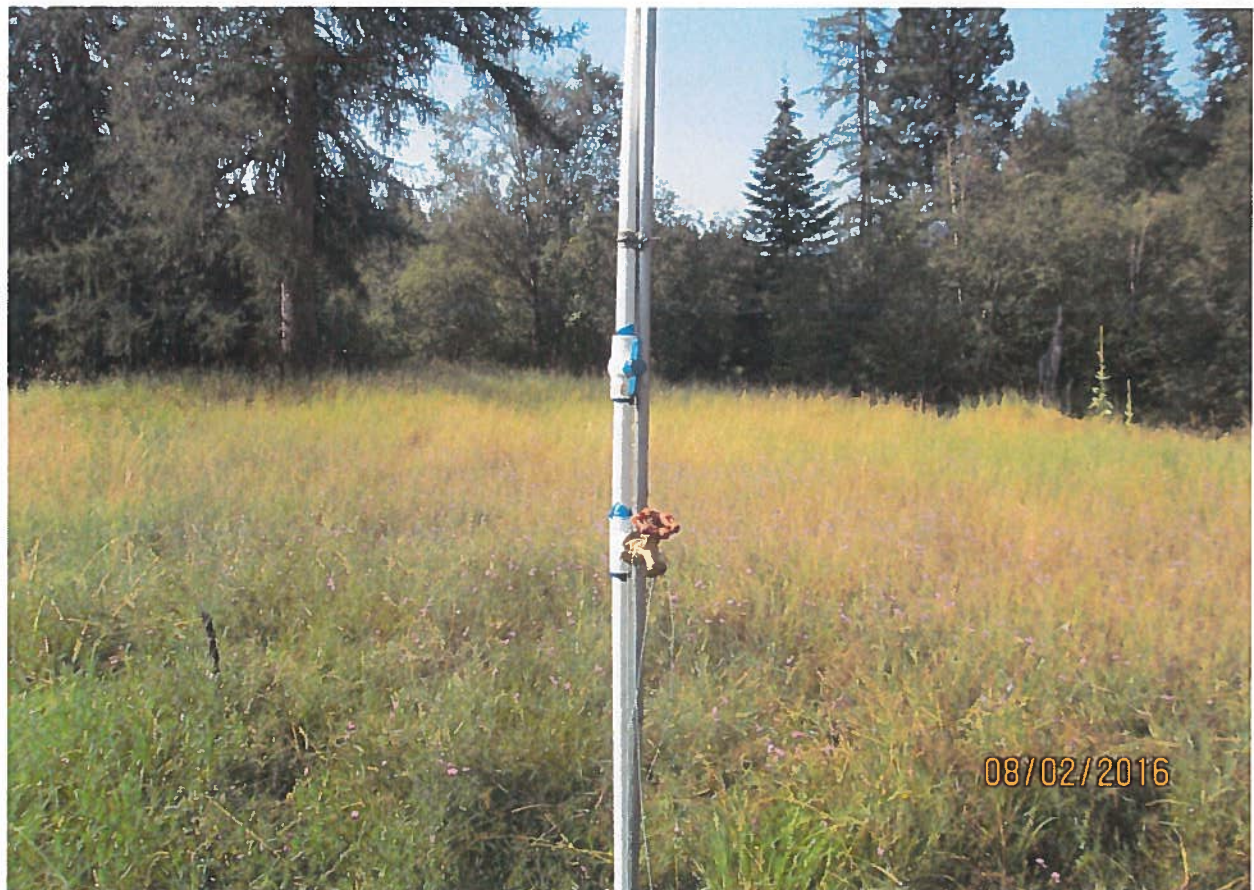
Additional hose connection at base of PVC pole.
