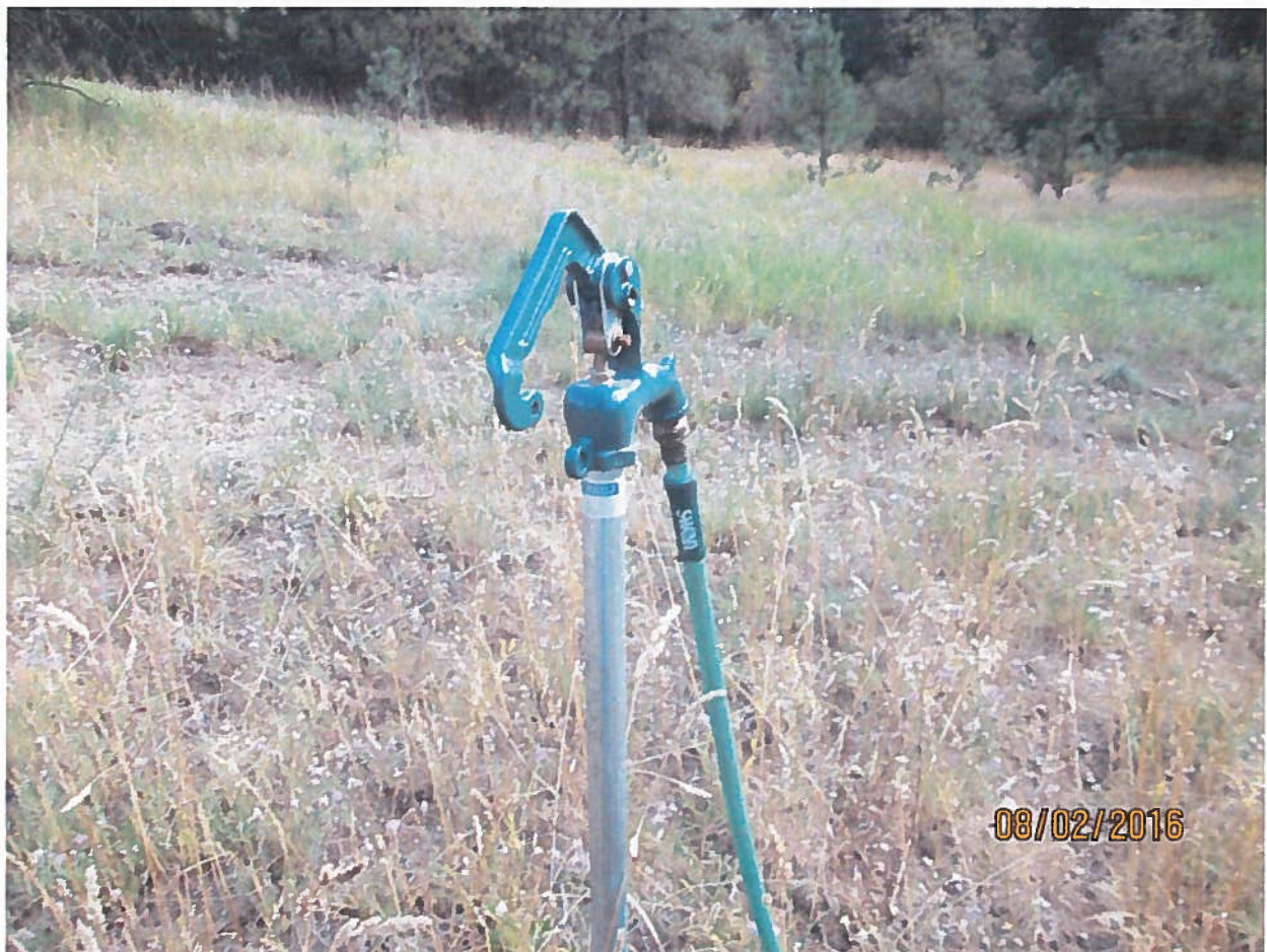
Frost free hydrant with hose.
