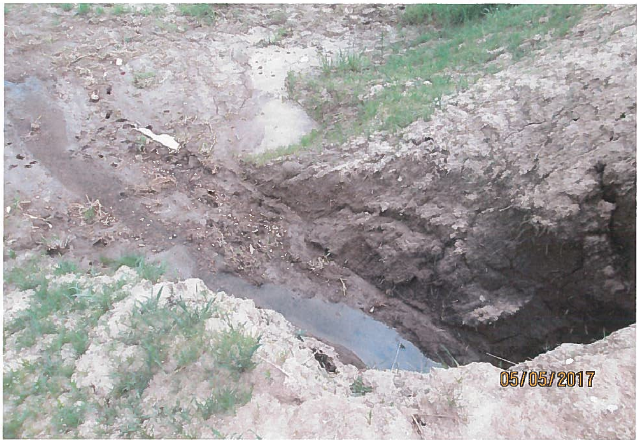
View downstream of dam with debris washout from dam.
