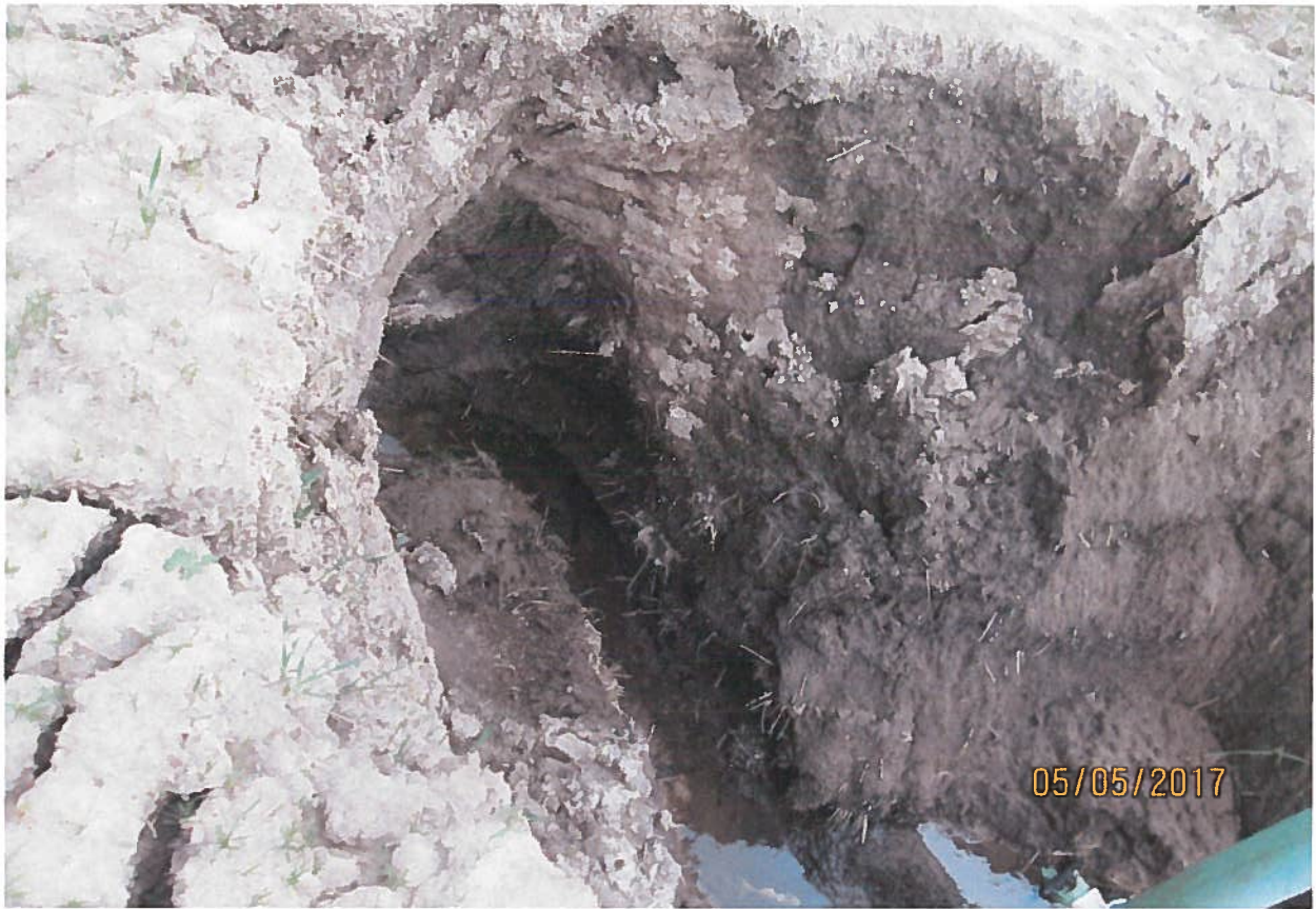
View of hole in dam after washout.
