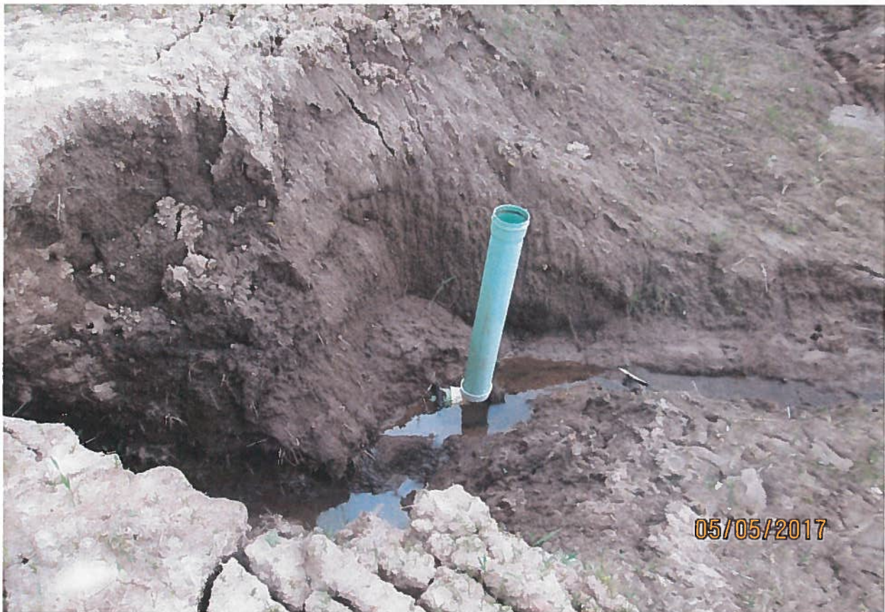
12 inch overflow pipe.
