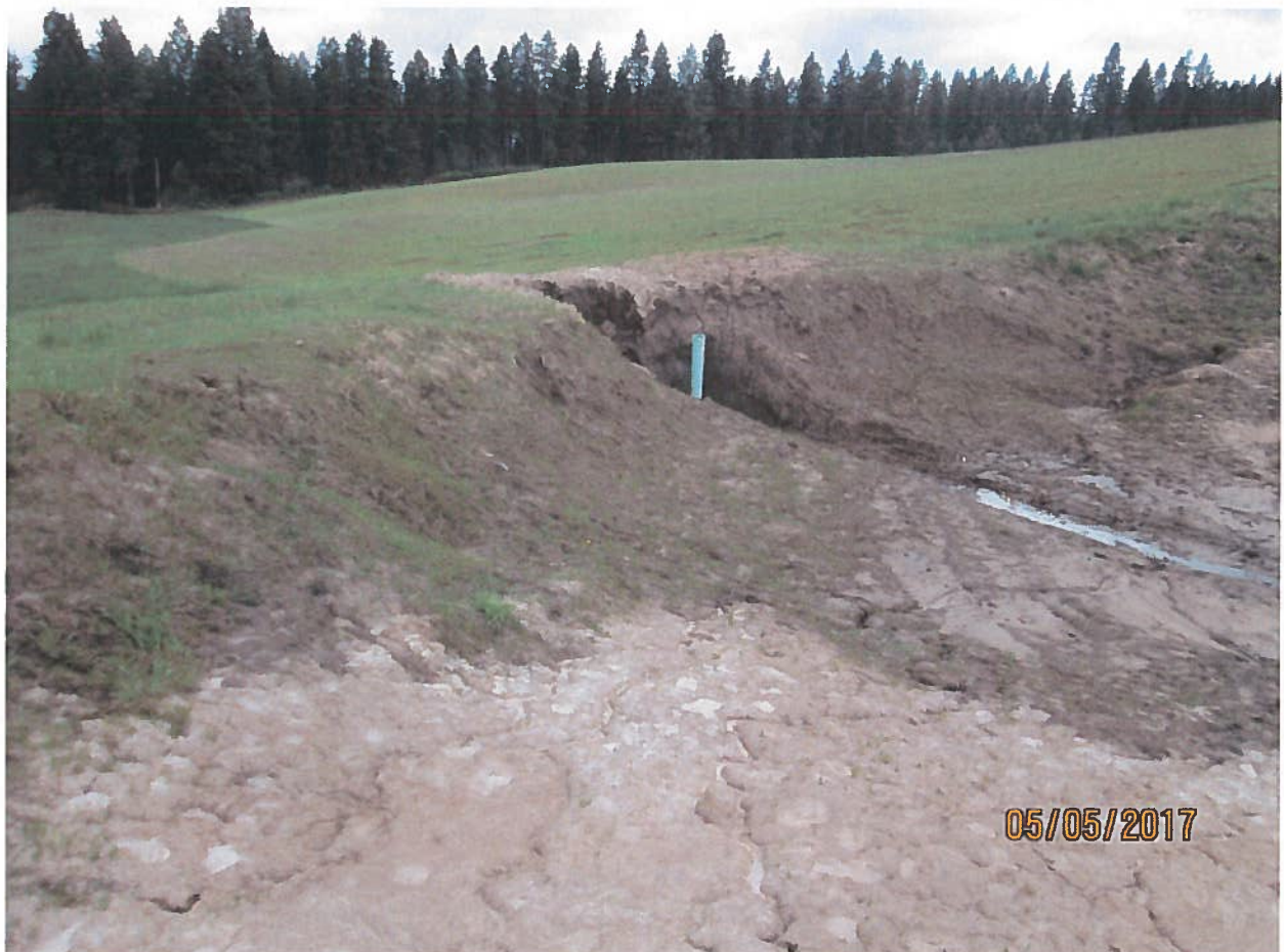
View of dam. Applicant said the dam washes out each year and he hasn't found a good way to keep it there.
