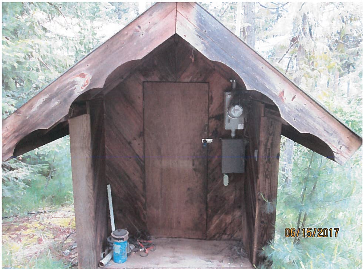
Well house over hand dug well.
