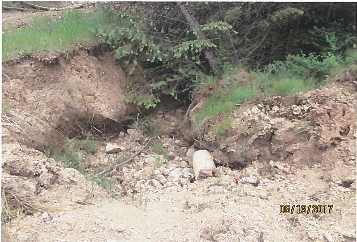
View downstream from dam. Culvert washed out this spring and had been replaced by applicant.
